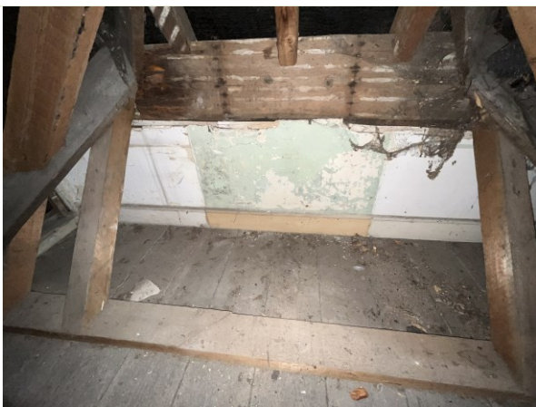
Scattered bat droppings in the topmost loft void
