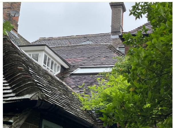
There are raised tiles throughout the roof
