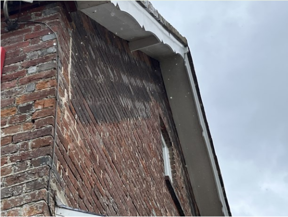
Gap behind the gable end soffit
