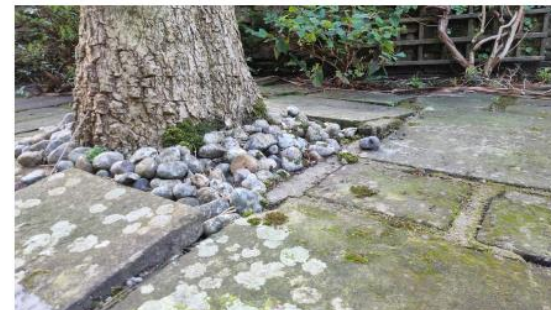
P3 SHOWING DAMAGE TO THE COURTYARD HOUSE WALL SIDE
