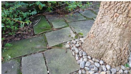
P1 SHOWING DAMAGE TO THE COURTYARD AND ENCROACHMENT ON STREET WALL SOUTH SIDE
