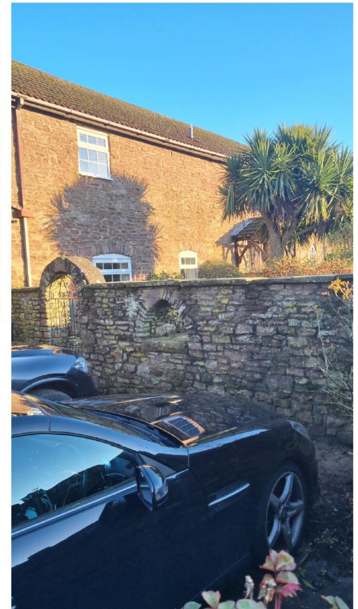
P6 LOOKING SOUTH EAST NOTE: SHADOW FROM THIS TREE PREVENTS LIGHT FROM ENTERING THE KITCHEN
