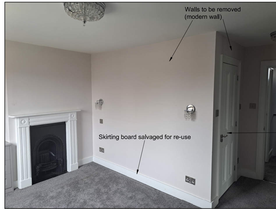
VIEW A: View of en-suite wall from bedroom (door to be salvaged for re-use in new shower room wall)
