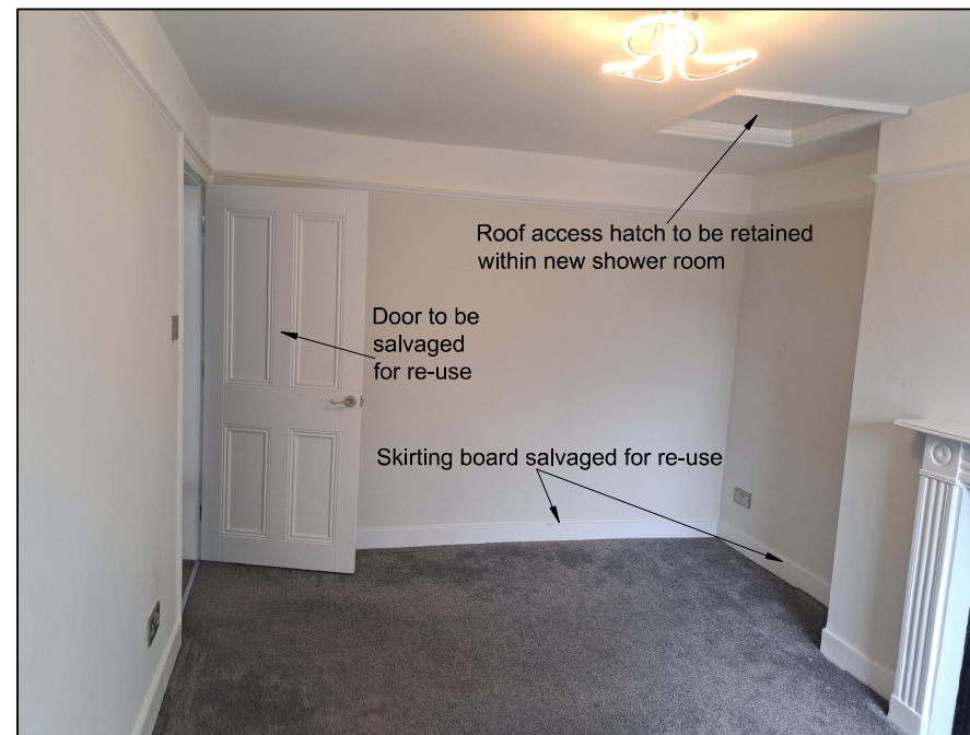
VIEW C: View of area where new ensuite shower room is to be formed
