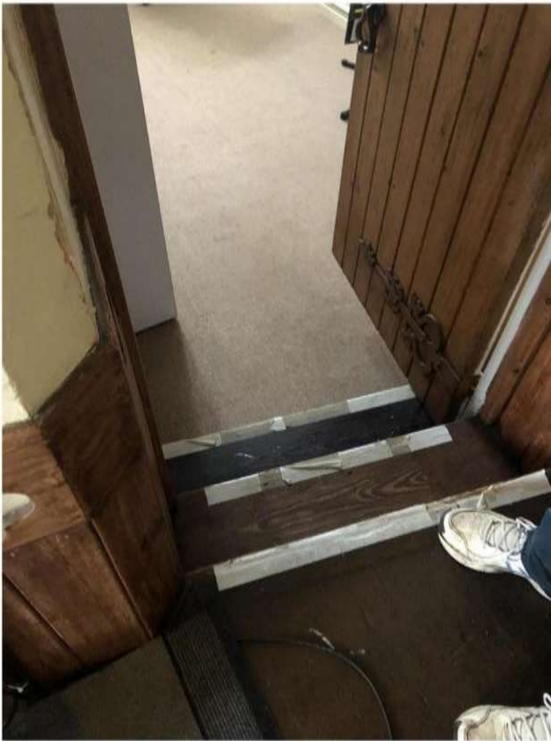
iii) vestry door from stage, showing how the door is set to the original floor height.
