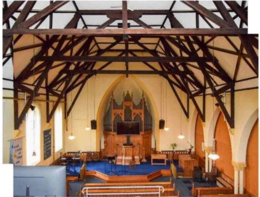
ii) Looking west - note insertion of screens much reducing natural light and strengthening of roof structure with the insertion of double collars bolted to either side of original timbers
