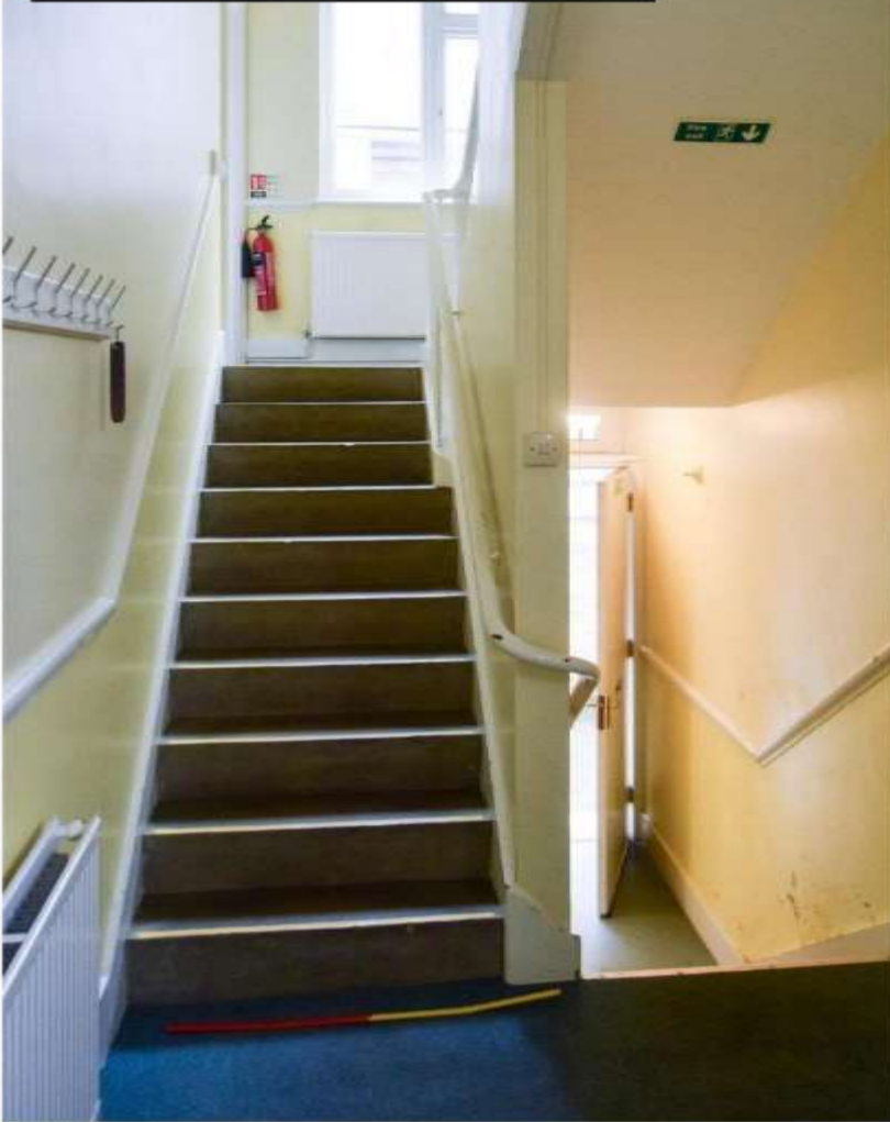
i) the classroom block is accessed (to right) from half a storey below its ground floor rooms via a concrete stair.
