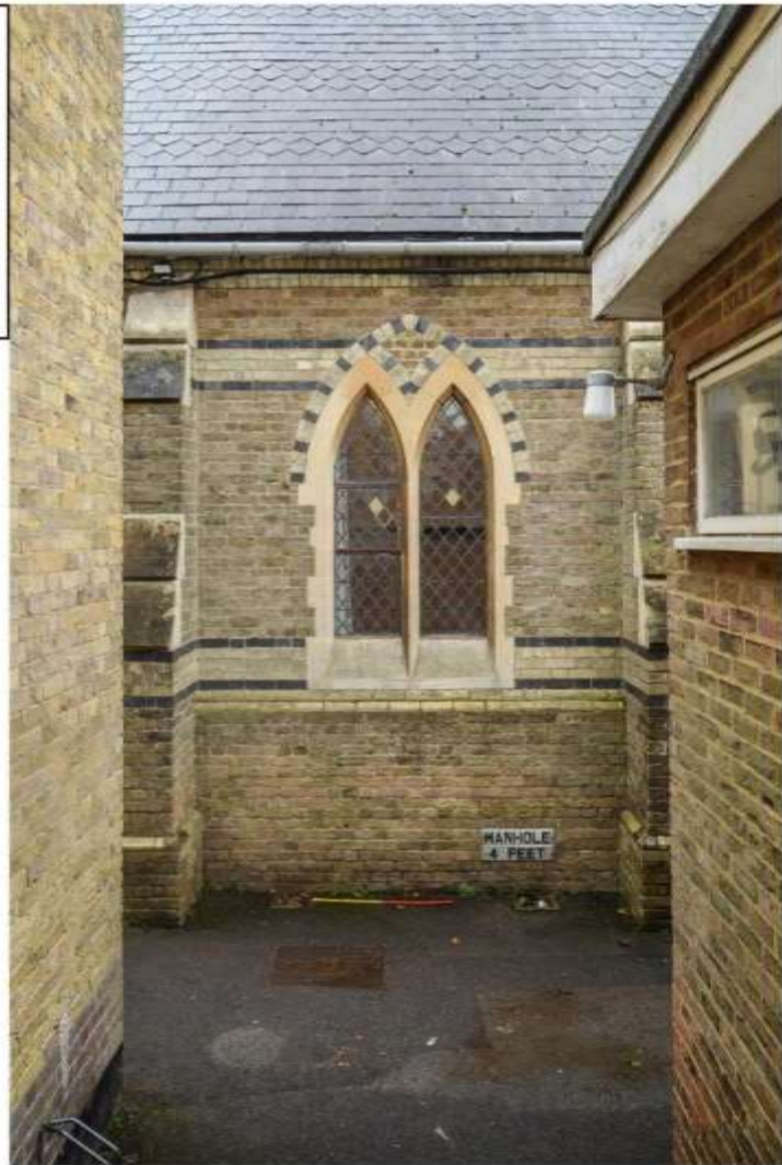
iv) smaller paired lancet of north elevation (schoolroom). note slating detail on roof
