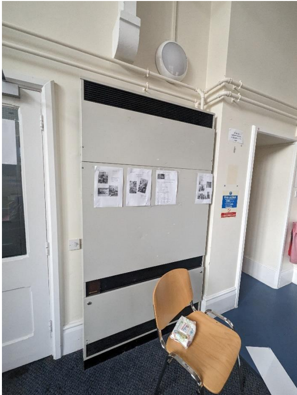
Figure 7 - Current heating unit
