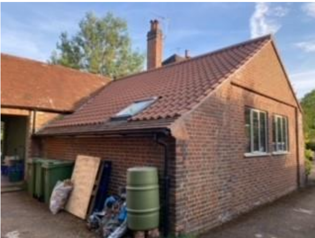
Family room side elevation (note lower pitch of new roof not matching house)
