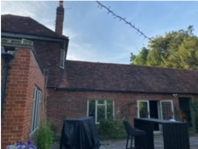
Rear elevation door head height to be reinstated
