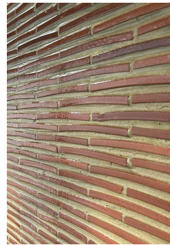
Wall constructed from creasing tiles, chosen to reference the tile detail to existing window openings
