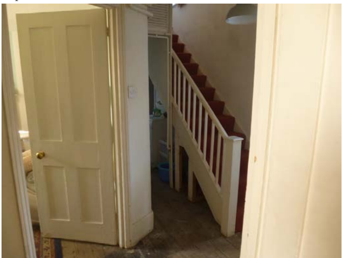
Figure 6 Basement staircase not spindles and hand rail/newel are recent. It is proposed to partition this off to create the annexe.
