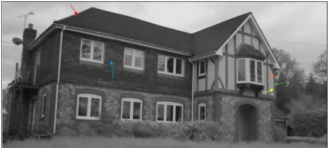
Figure 2. bat emergences from the eastern elevation during the first survey on 9 th May. Red arrow two bats, blue arrow three bats, orange arrow 1 bat, green arrow 10 bats, yellow arrow 7 bats.
