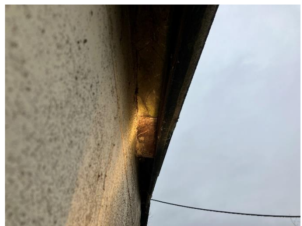
Photo 16: Large gap between barge boards and walls of Building 2 – not suitable for crevice dwelling bats
