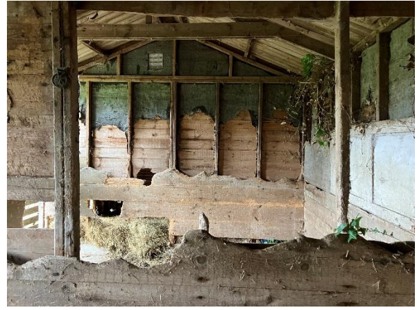
Photo 30: Internal view of Building 5, with chewed lower wall sections
