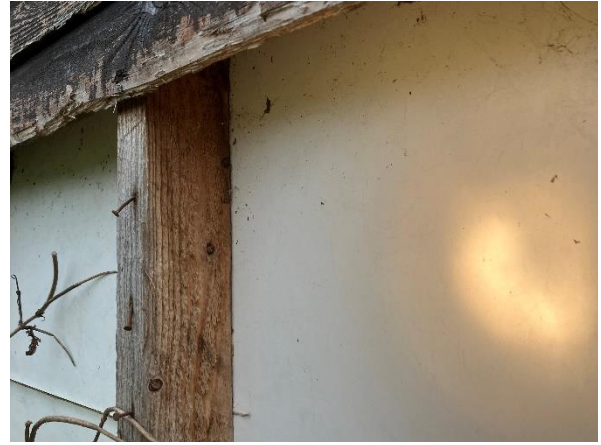
Photo 26: Slippery plastic surface of internal wall lining
