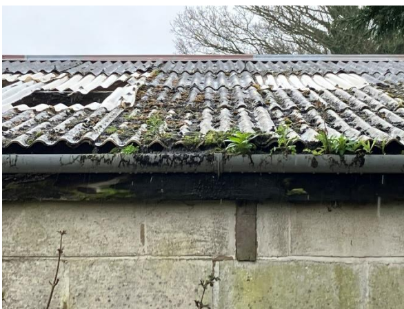
Photo 15: Building 2 roof structure – fibreboard sheets, broken Perspex sheets and a metal ridge covering
