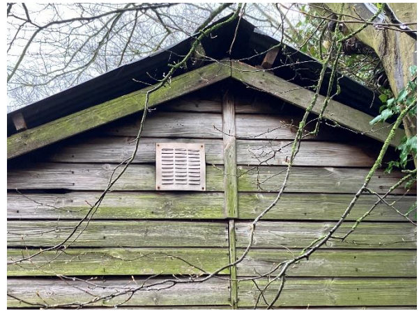
Photo 32: Large gap between tin roof covering and wooden sarking beneath
