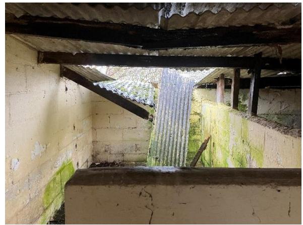
Photo 20: Internal view of Building 3, south western end, with partially collapsed roof
