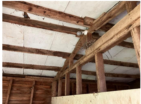
Photo 28: Roof structure of B5, with bird nest on beam
