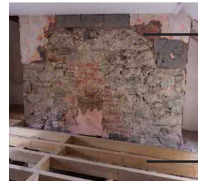
South gable traditional stone work chimney breast patched up with concrete blocks and bricks.
