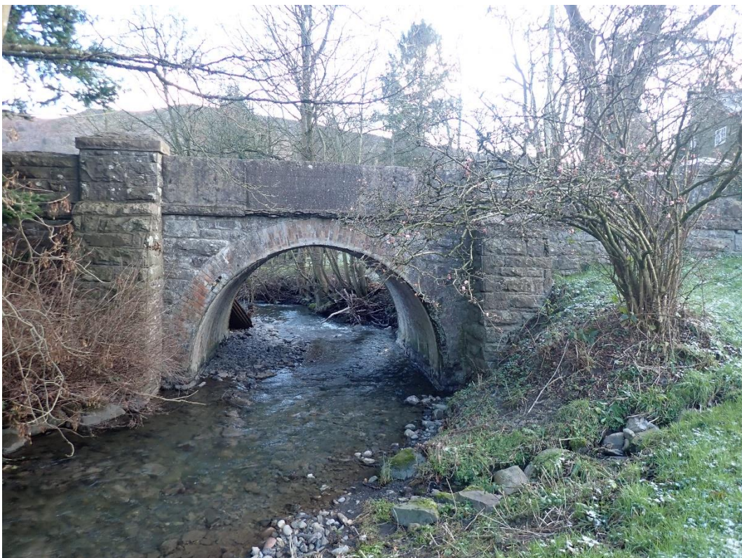
Photo 8. View of the road bridge. This structure did not have any potential for bat roosts.
