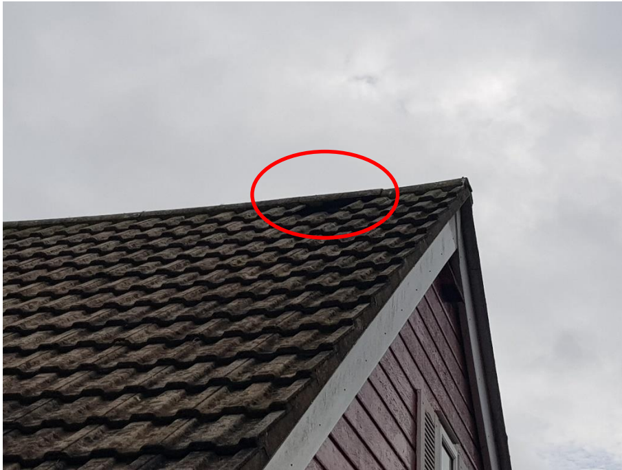
Plate 5 - Missing tile from house roof (B1), potential roosting feature for bats and birds
