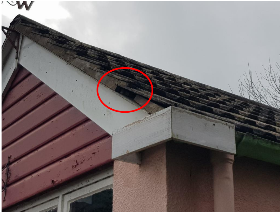
Plate 7 - Gap in the mortar in outbuilding (B2), potential roosting feature for bats and birds
