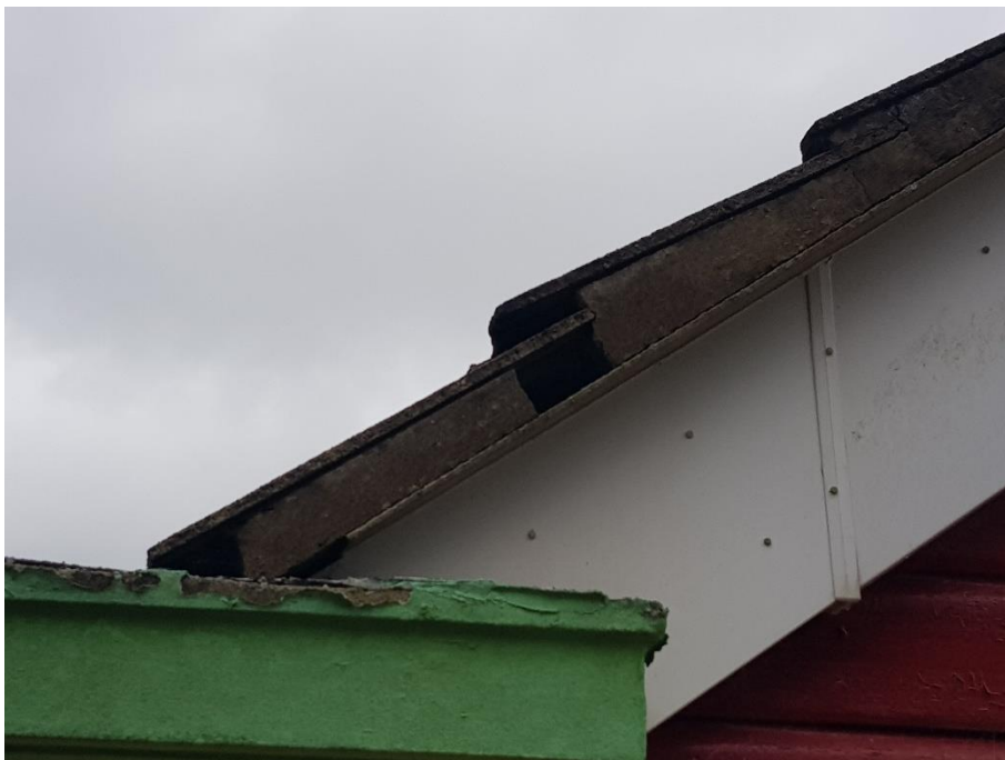
Plate 6 - Gap in the mortar in house (B1), potential roosting feature for bats and birds
