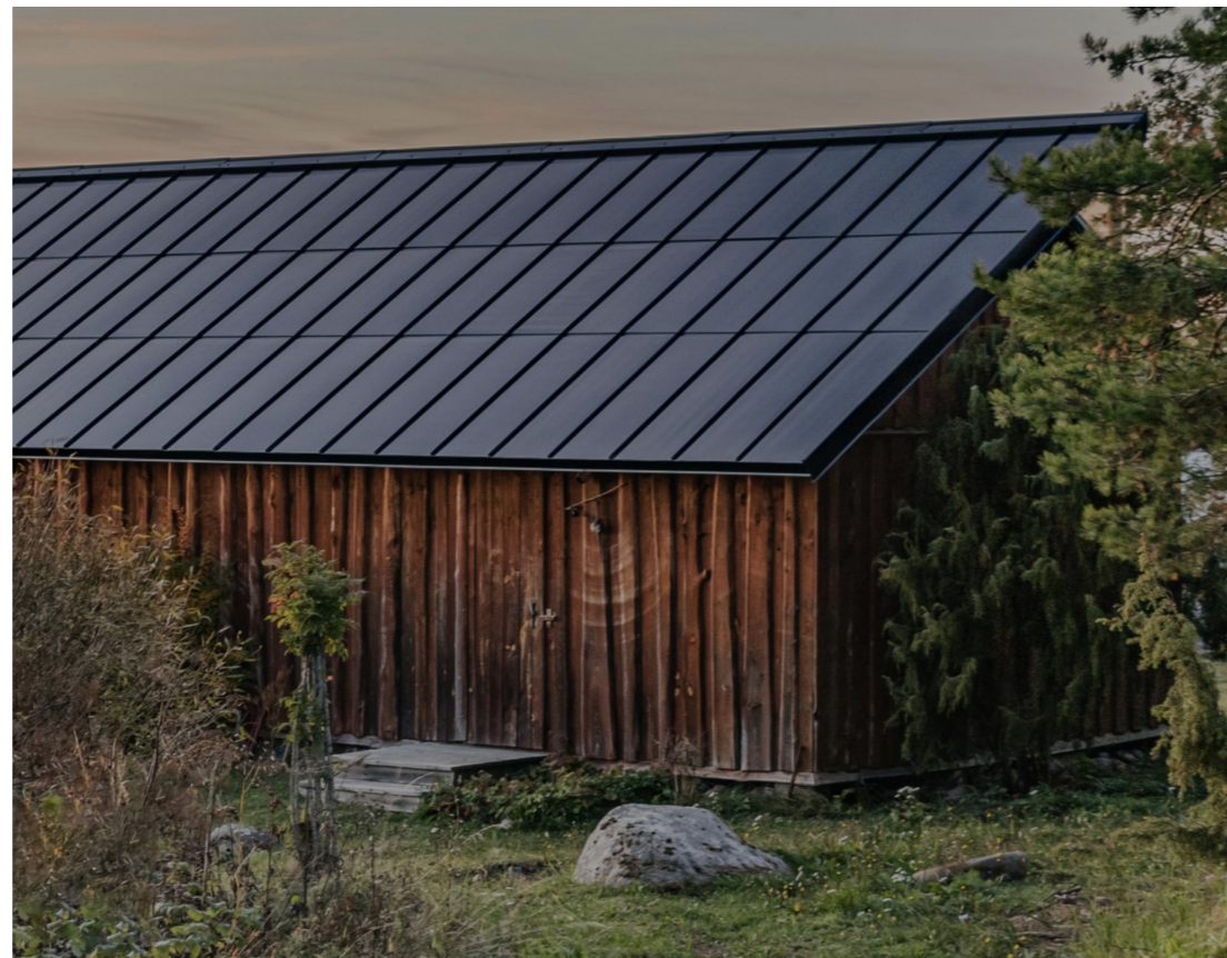
PV panels blended into metal roofing
