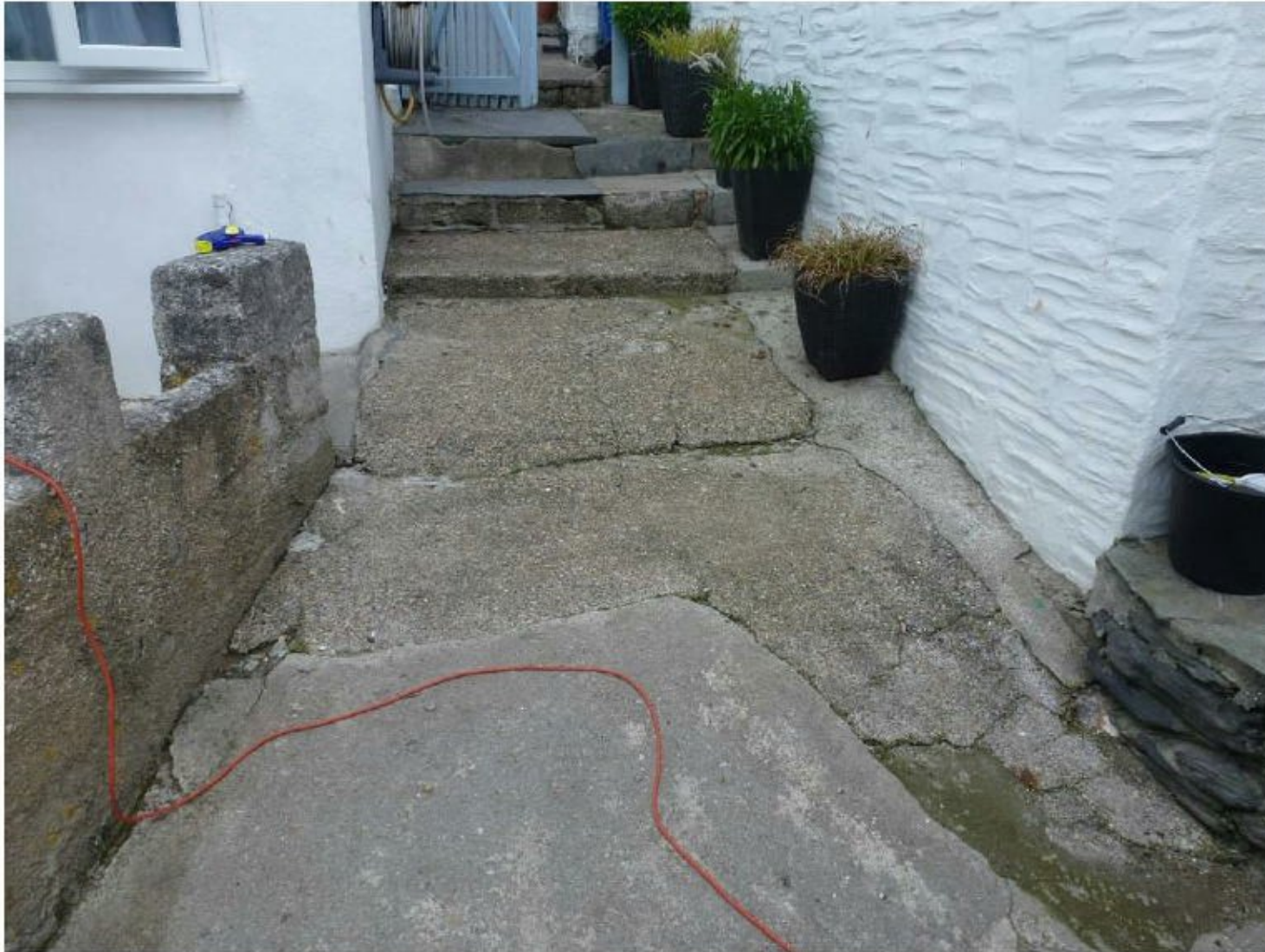
Photograph 4 – Old footway cracking to front and right of main bungalow
