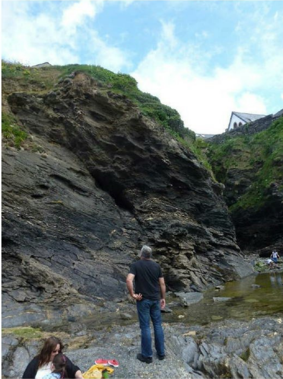
Photograph 8 - Main rock outcrop under property looking up (note tip of roof of timber shed to left side)
