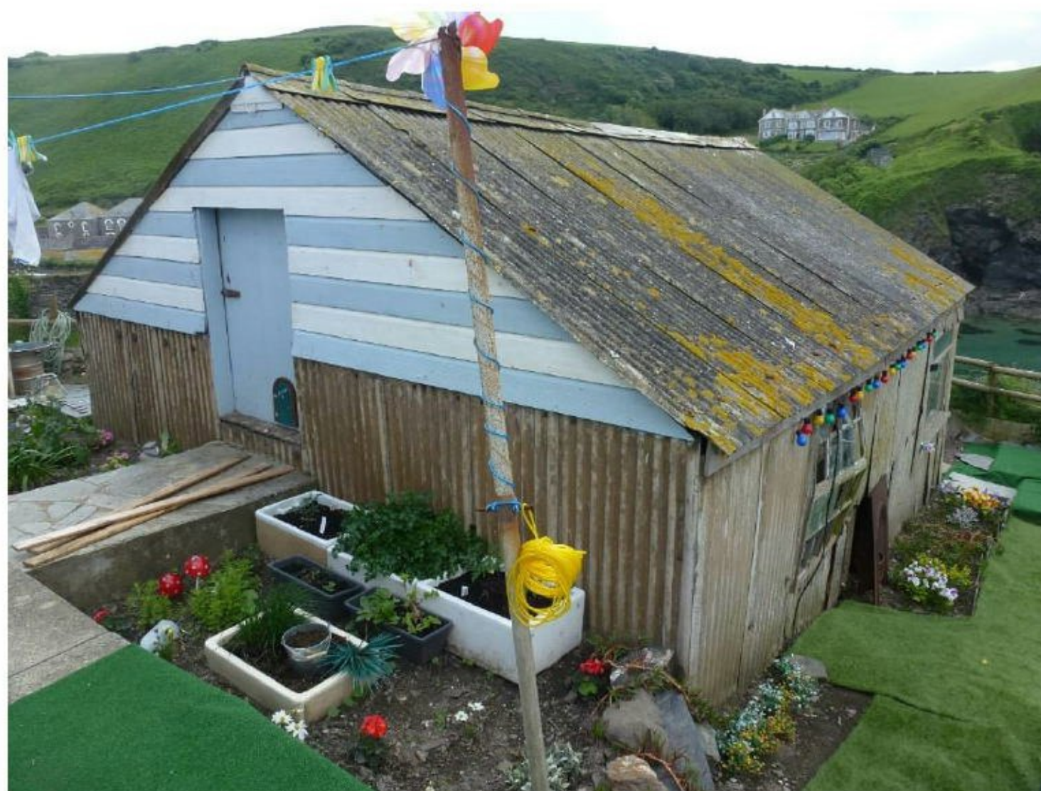
Photograph 3 – Crack to southern elevation to junction of extension
