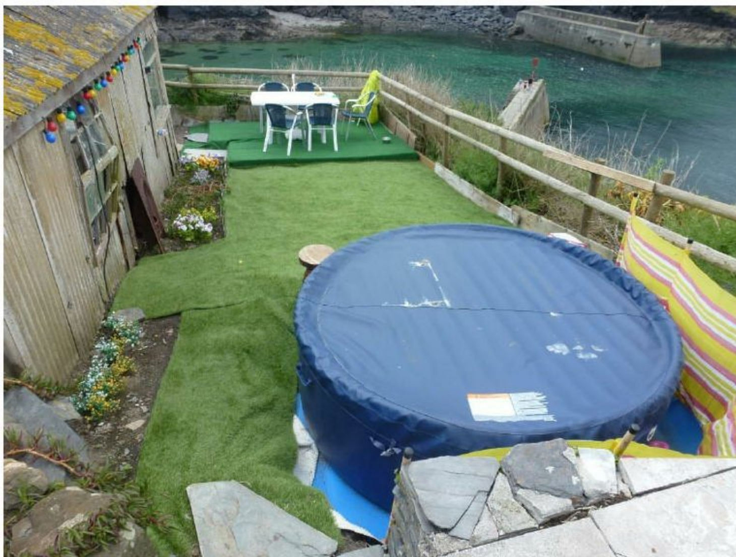
Photograph 7 – Fencing around north of site showing signs of age and wear and tear
