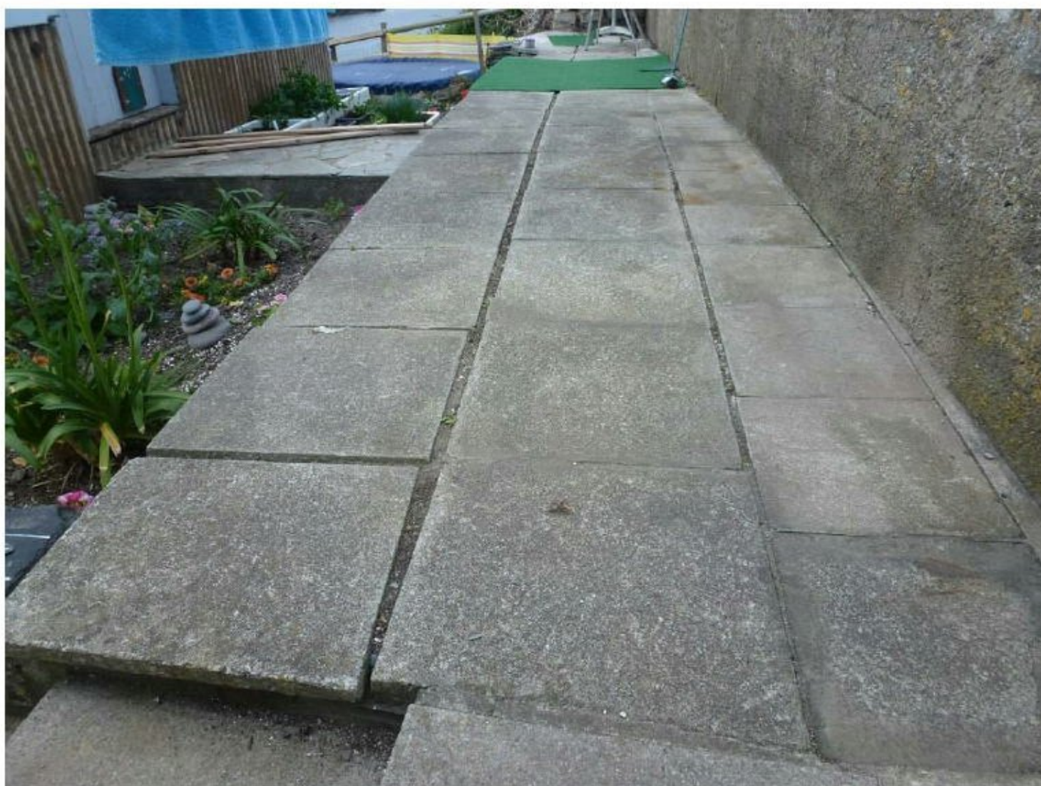
Photograph 6 – Footway in front of internal garden wall showing some signs of old lateral movement towards the cliff
