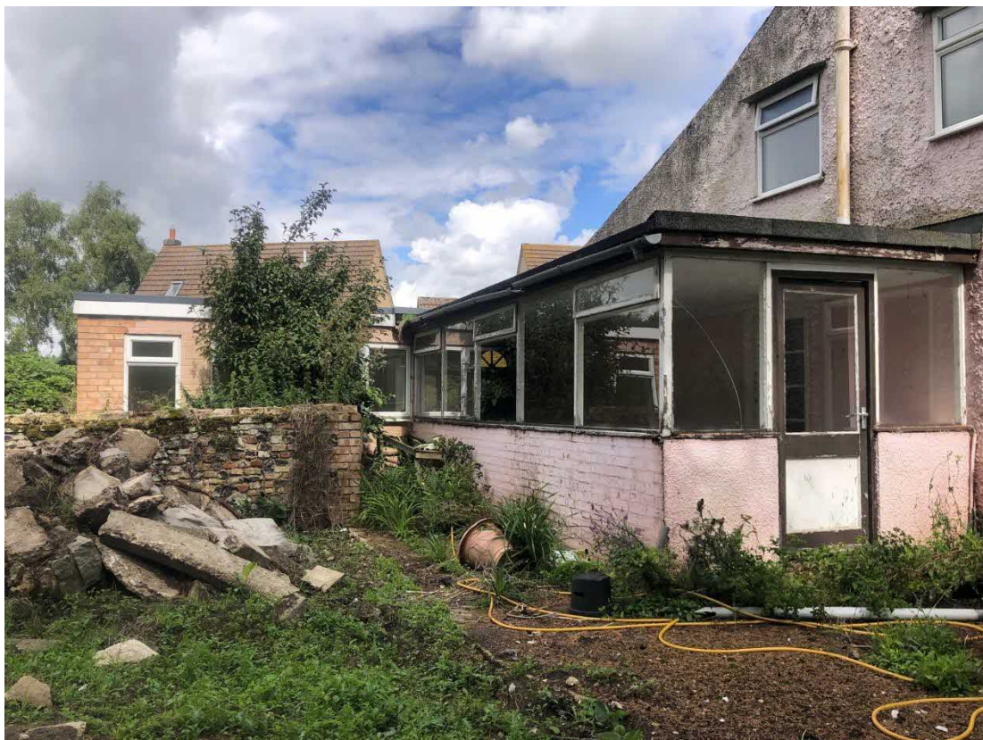
Photo 11, south and east aspects of two extensions on western aspect of building one, looking north.
