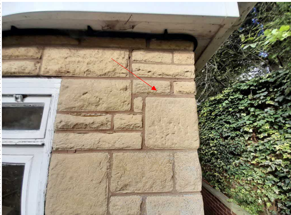
Plate 7. Stepped cracking front elevation of single-storey addition.
