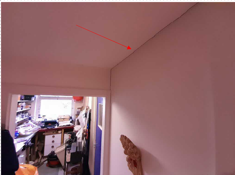
Plate 16. Cracking to junction between single-storey addition and main property.
