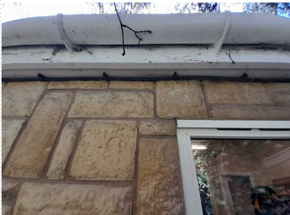
Plate 9. Stepped cracking above single-storey right-hand elevation window (garage/workshop).
