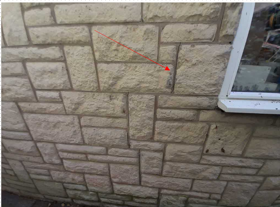
Plate 8. Stepped cracking to right-hand elevation of single-storey addition (garage/workshop).
