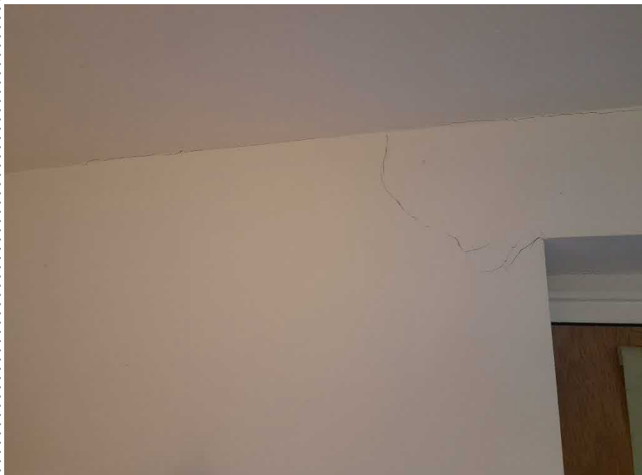
Plate 15. Diagonal crack above external door opening.
