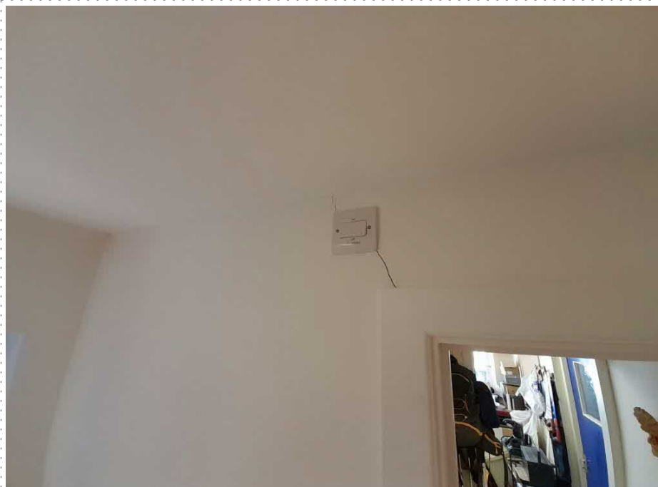
Plate 18. Diagonal cracking above second kitchen door.
