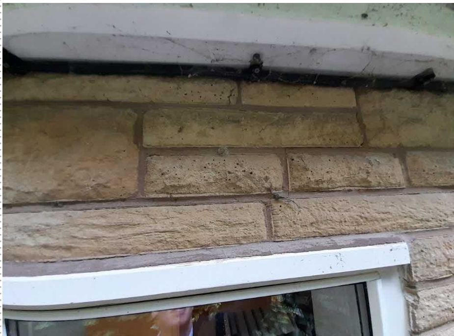
Plate 11. Stepped cracking above single-storey right-hand elevation window (utility).
