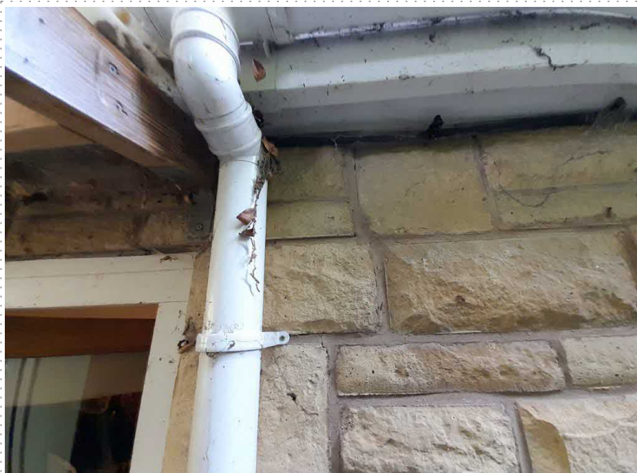
Plate 12. Vertical cracking to right-side single-storey addition external door opening.
