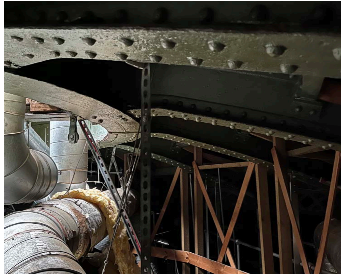
Image top left: aerial view of existing cupola Image top right: internal view of existing cupola Image bottom left: existing roof structure and sarking Image bottom right: general condition of existing roof structure
