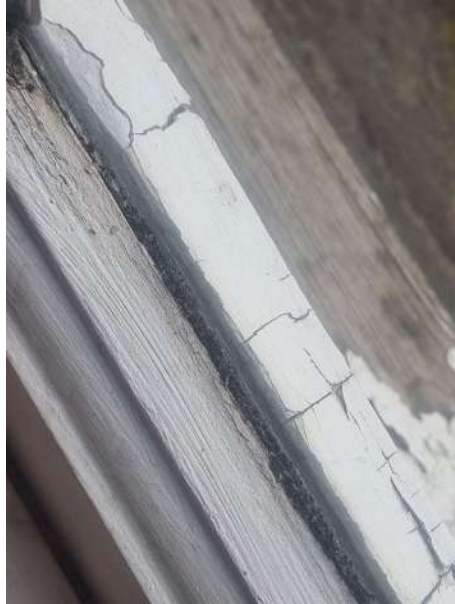
Broken exterior putty is allowing water to enter the woodwork
