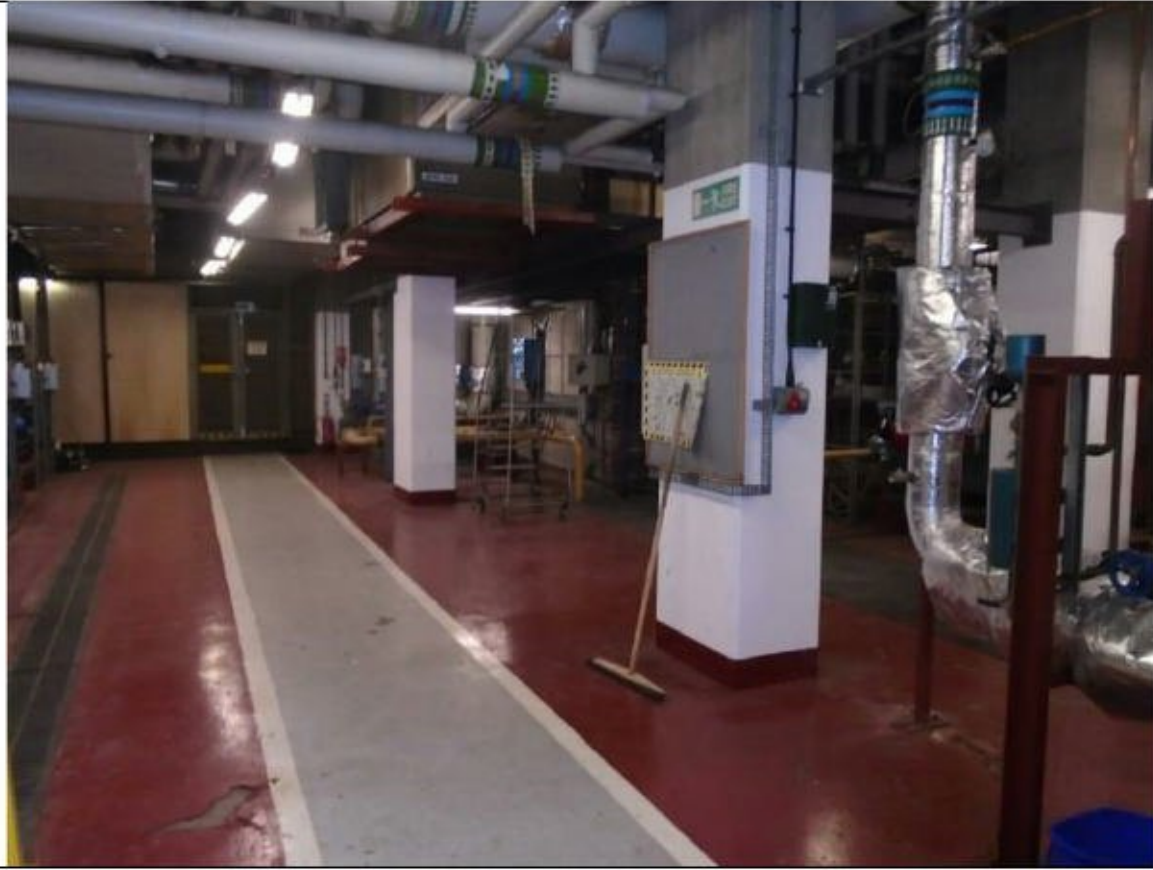
Photograph 1: Example of Internal plant room
