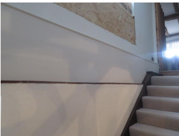
Boxing (above row of tiles) to accommodate redundant radiator pipes to be removed
