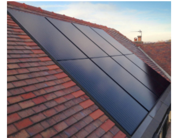
Photovoltaics to roof
