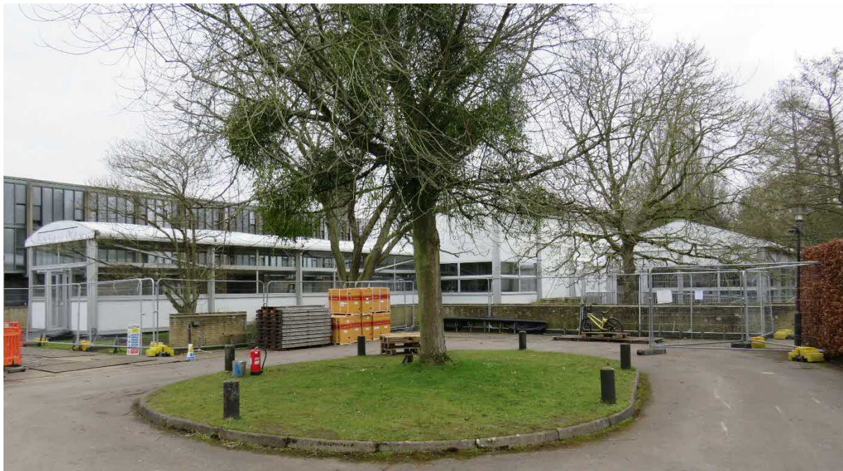
Lecture theatre marquee under construction, viewed from the turning circle at the south end of the access drive. Further photographs are included with the submitted drawings
