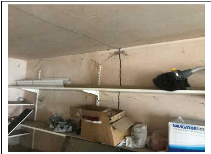
Internal crack in the partition wall between garage/office and ceiling
