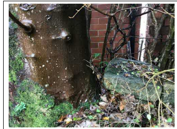
Proximity of the sycamore tree to left-hand side wall.
