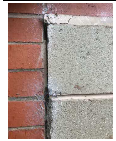
Cracking over garage door (top left-hand corner)
