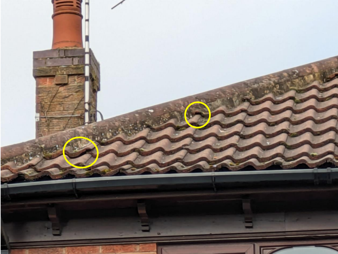
Photograph 7: The southern aspect of the roof showing the lifted tile.
