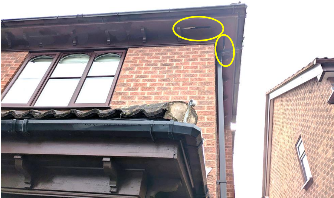
Photograph 8: The missing mesh on the vents into the soffits.
