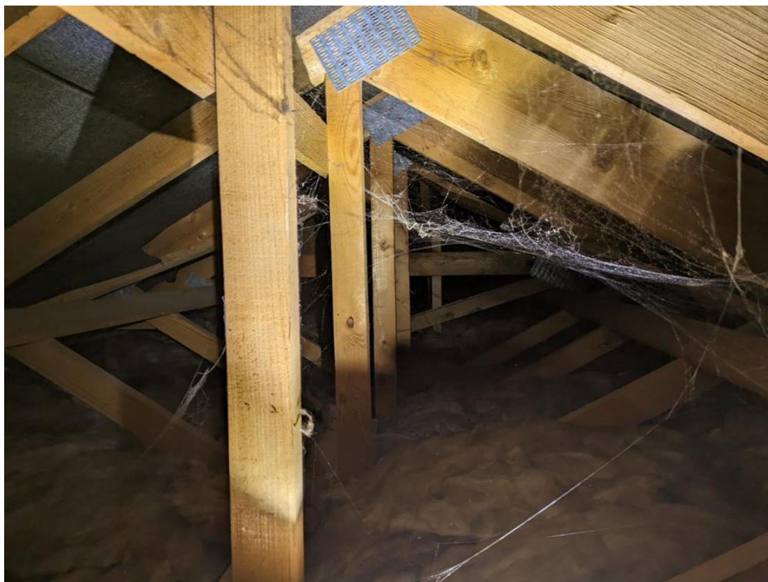
Photograph 6: The internal roof void showing dense cobwebs.
