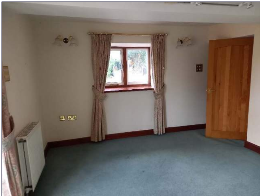
Plate 25: View looking north-east showing the northern room on the ground floor of the original house; access to the conservatory is to left of photograph
