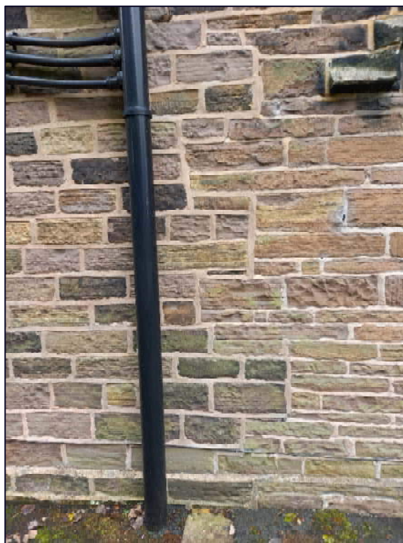
Plate 13: North-east elevation of Rotherham Top Farm showing the construction break between the 17th century fabric (right) and late 20th century extension (left)
