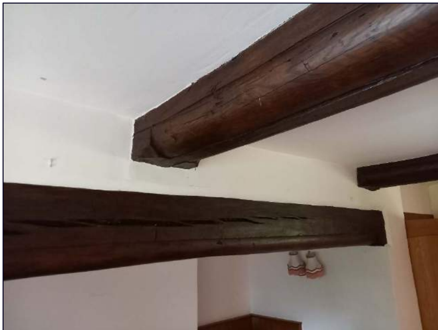
Plate 23: Detail of the bressummer (spanning the fireplace), and the two beams with ovolo moulding and chamfer stops, ground floor of original house
