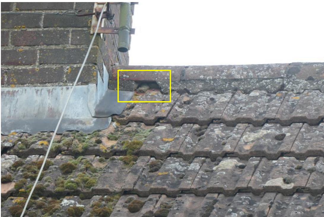
Photo 13 , example of gaps around the chimney.
