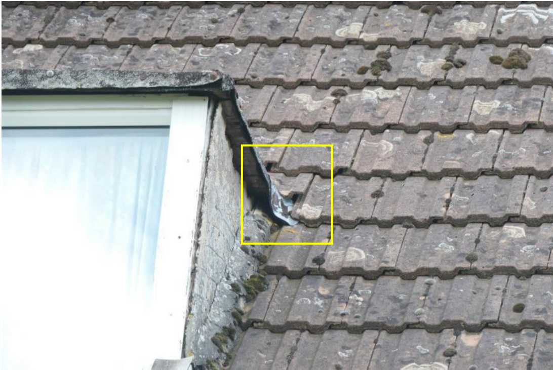
Photo 14 , example of gaps around dormer windows.
