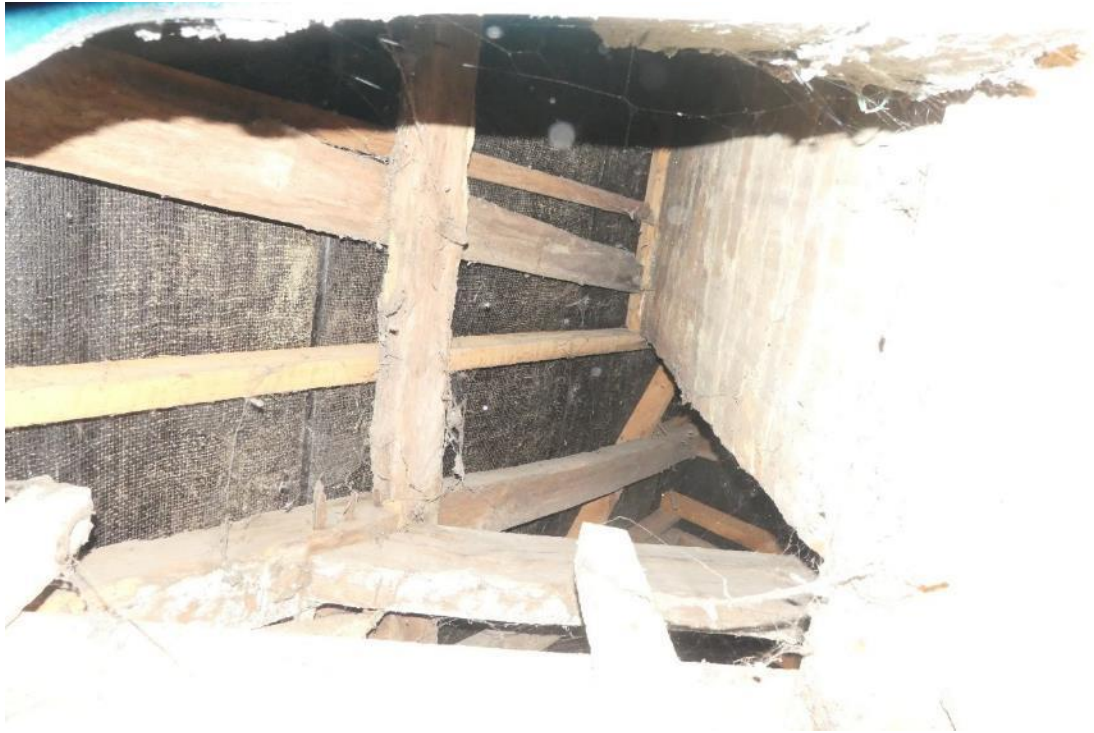
Photo 17 , gaps around chimney which allow access into the main loft space from the living areas.
