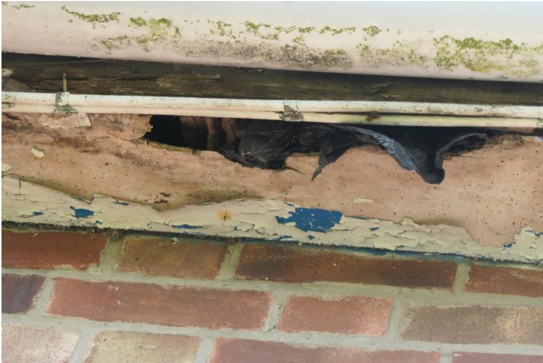
Photo 12 , example of holes in the soffits of the building.
