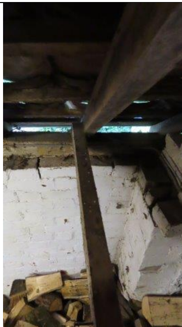
Gaps under eaves of logstore.
