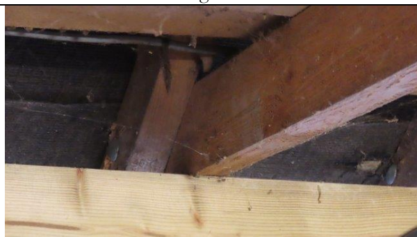
Close-fitting timber joints, which were typical throughout the interior of the building.
