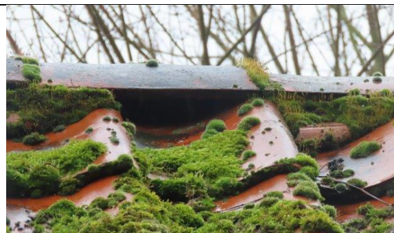
Gaps in mortar between ridge and pan tiles.
