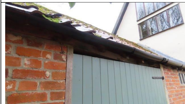
Gap above doorway on western elevation.
