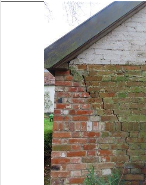
Extensive cracks running across northern elevation.
