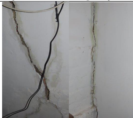
Cracks caused by ground subsidence, interior walls.
