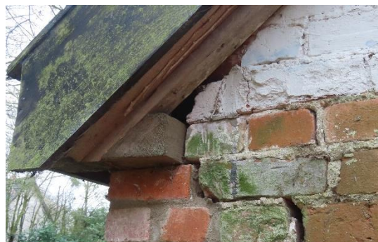
Cracks in the brickwork of northern elevation of extension.
