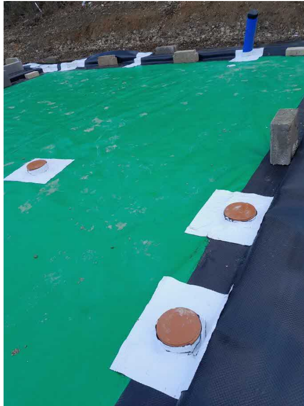
03 C8785E 23.01.23 Plot 32 Service Entry Ducts
