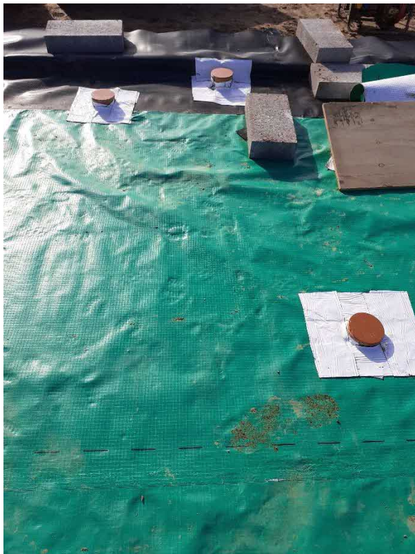
04 C8585E 29.09.22 Plot 51 Service Entry Ducts
