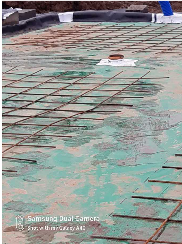
03 C8785E 29.03.23 Plot 55 Corners and Service Entry Duct (client photo)
