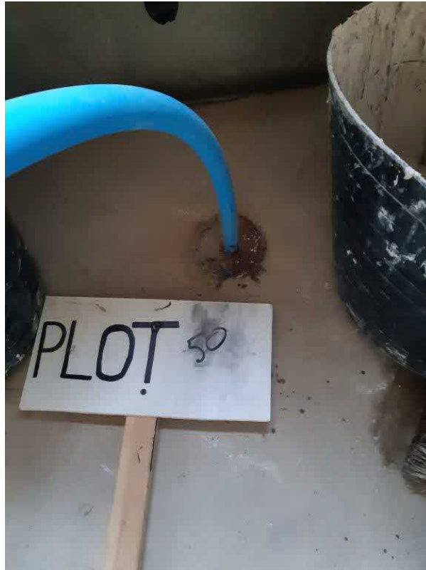
05 C8785E 10.11.23 Plot 50 Service Entry Seal (client photo)
