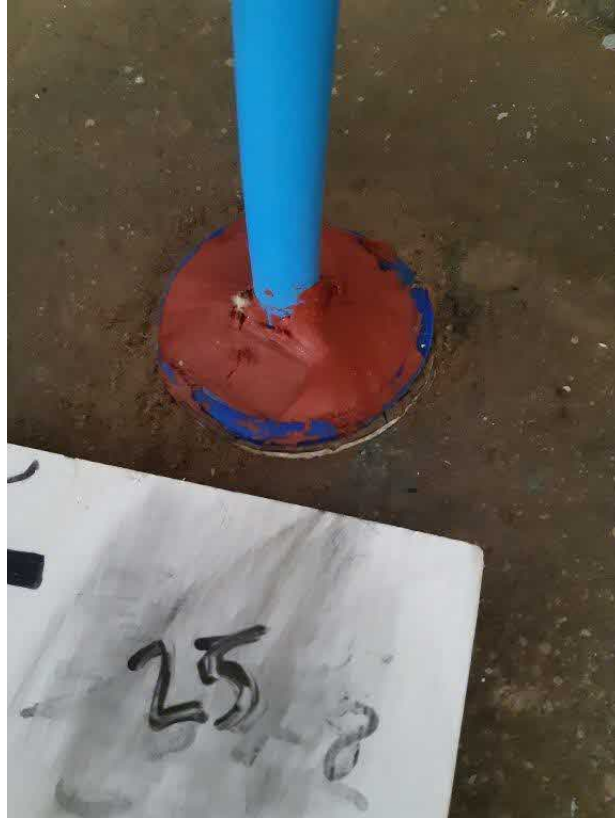
03 C8785E 15.09.23 Plot 25 Service Entry Seal (client photo)
