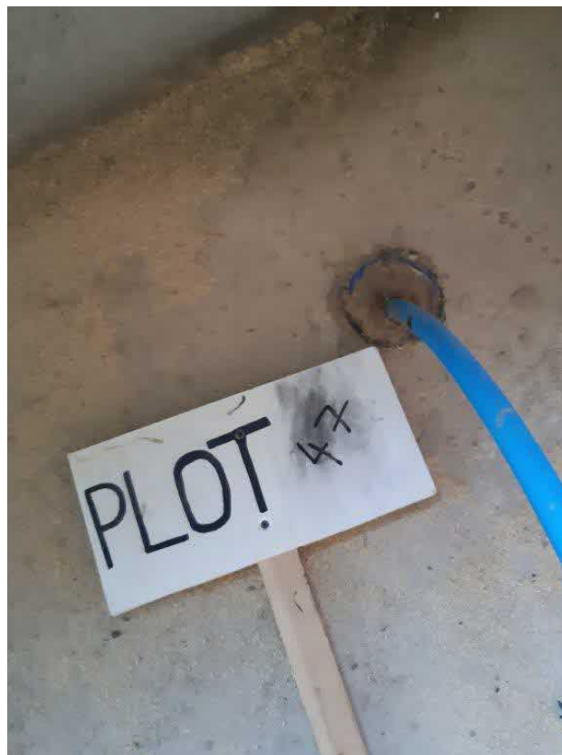
02 C8785E 10.11.23 Plot 47 Service Entry Seal (client photo)
