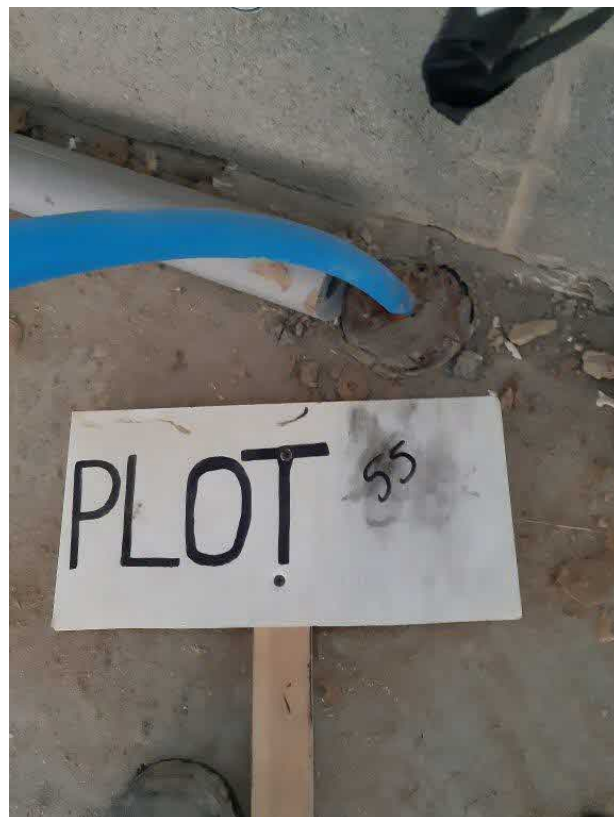
10 C8785E 10.11.23 Plot 55 Service Entry Seal (client photo)
