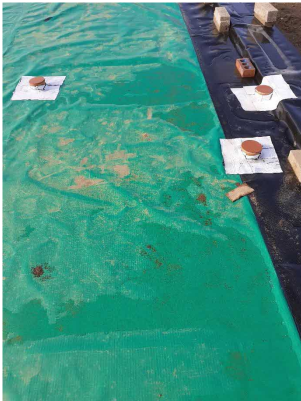
04 C8585E 29.09.22 Plot 47 Service Entry Ducts
