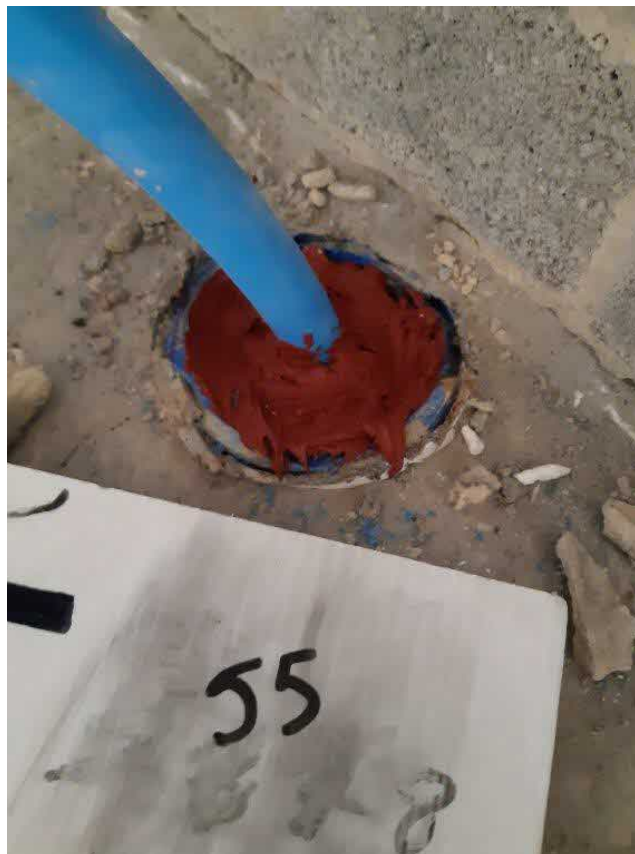
02 C8785E 15.09.23 Plot 55 Service Entry Seal (client photo)
