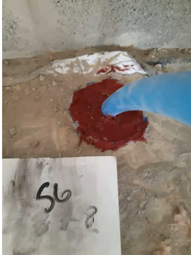
03 C8785E 15.09.23 Plot 56 Service Entry Seal (client photo)
