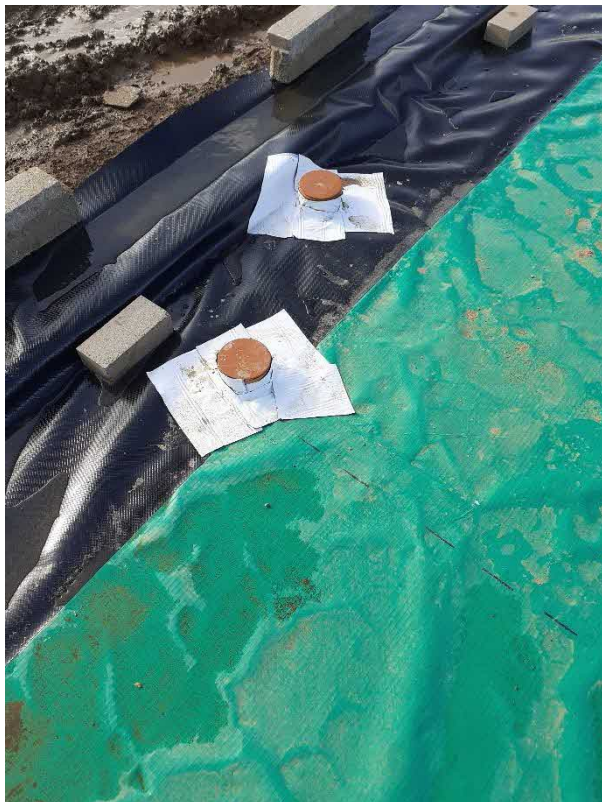
04 C8585E 29.09.22 Plot 48 Service Entry Ducts
