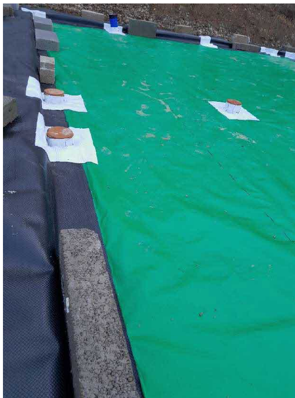
04 C8785E 23.01.23 Plot 31 Service Entry Ducts (client photo)
