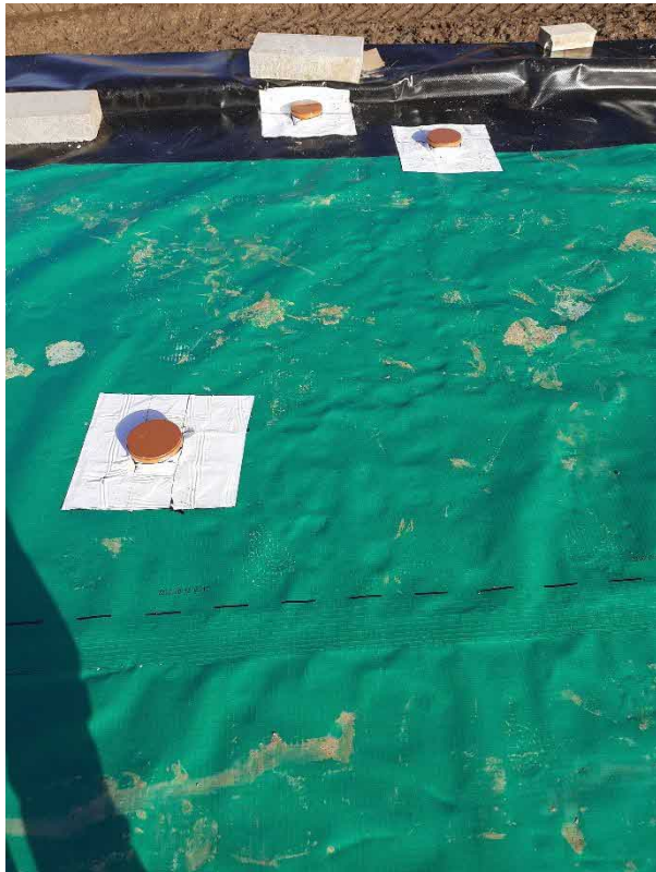
04 C8585E 29.09.22 Plot 49 Service Entry Ducts
