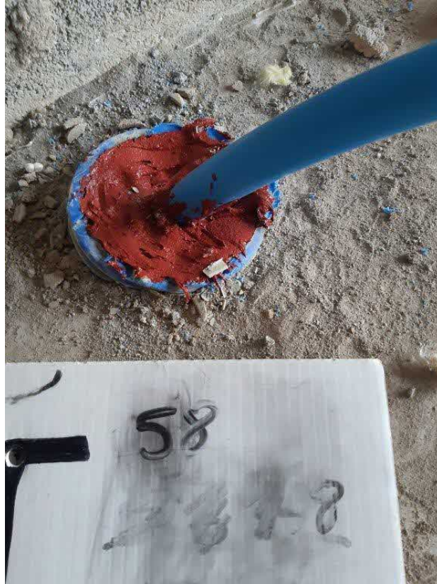
05 C8785E 15.09.23 Plot 58 Service Entry Seal (client photo)
