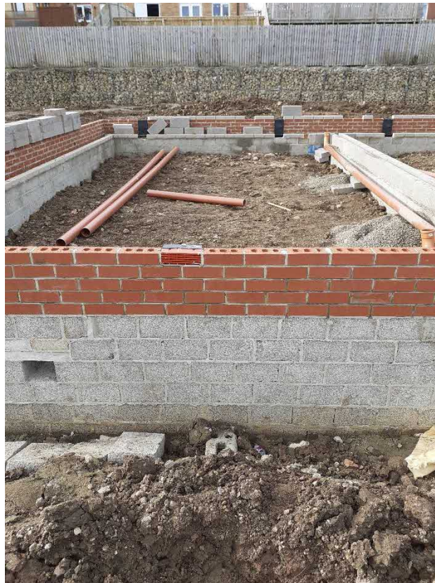
01 C8785E 20.02.23 Plot 25 Void Space (client photo)
