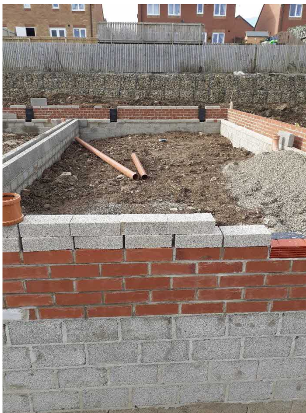
05 C8785E 20.02.23 Plot 25 Void Space (client photo)
