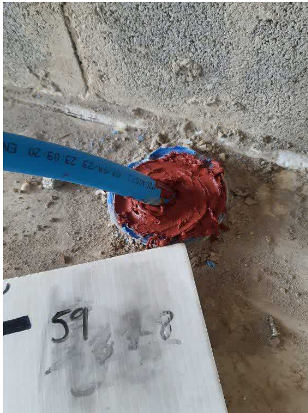
06 C8785E 15.09.23 Plot 59 Service Entry Seal (client photo)
