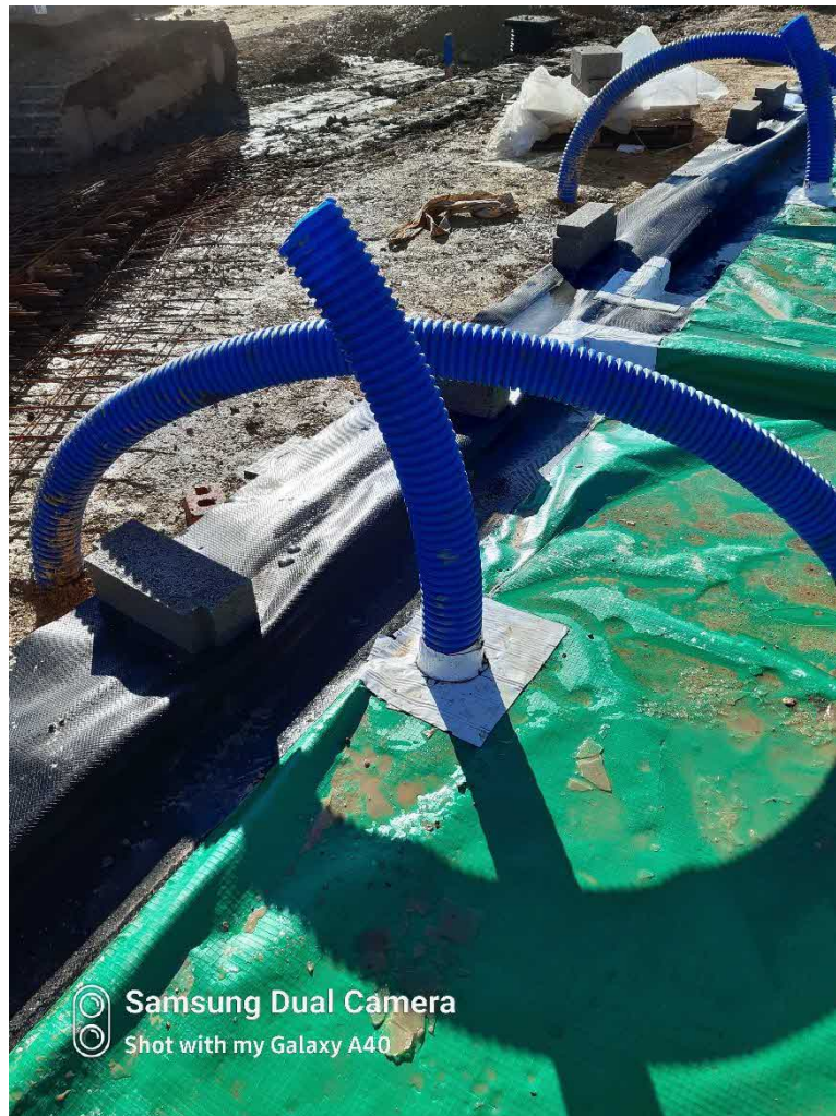
03 C8785E 03.04.23 Plot 23 and 24 Service Entry Ducts (client photo)
