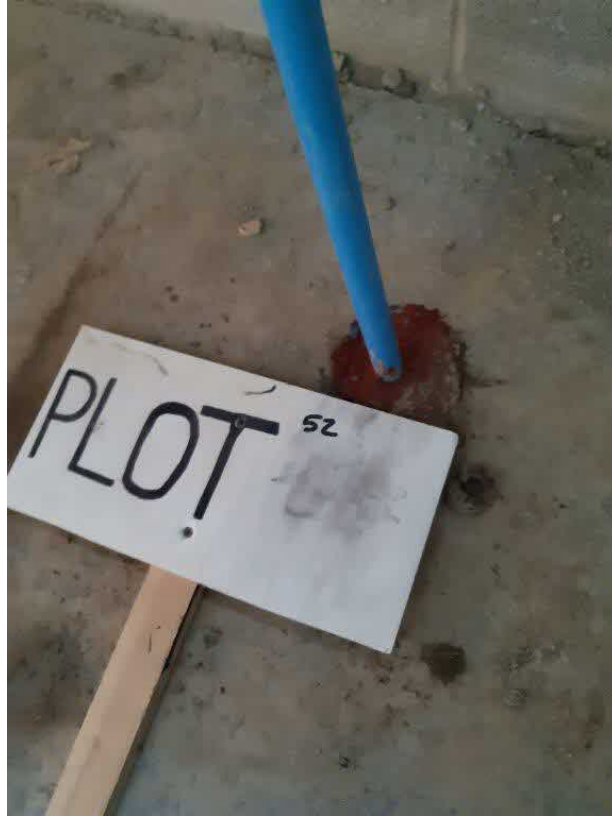
07 C8785E 10.11.23 Plot 52 Service Entry Seal (client photo)
