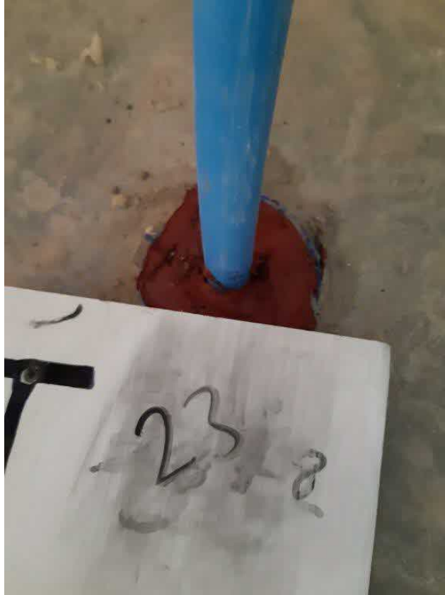
01 C8785E 15.09.23 Plot 23 Service Entry Seal (client photo)
