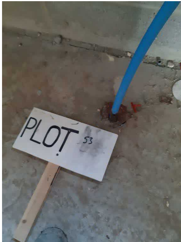
08 C8785E 10.11.23 Plot 53 Service Entry Seal (client photo)
