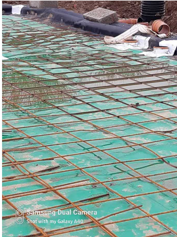
03 C8785E 29.03.23 Plot 54 Service Entry Ducts (client photo)
