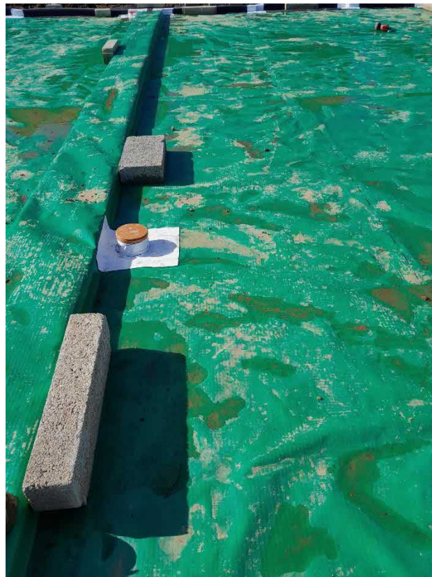
04 C8785E 07.03.23 Plot 25 Overview and Service Entry Duct (client photo)
