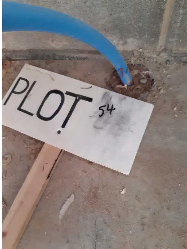
09 C8785E 10.11.23 Plot 54 Service Entry Seal (client photo)
