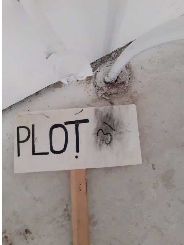
01 C8785E 10.11.23 Plot 31 Service Entry Seal (client photo)
