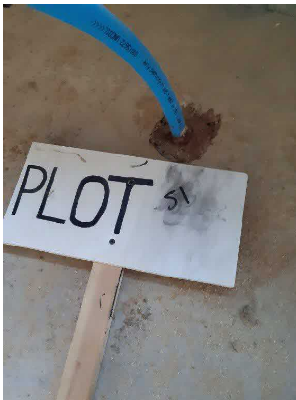
06 C8785E 10.11.23 Plot 51 Service Entry Seal (client photo)
