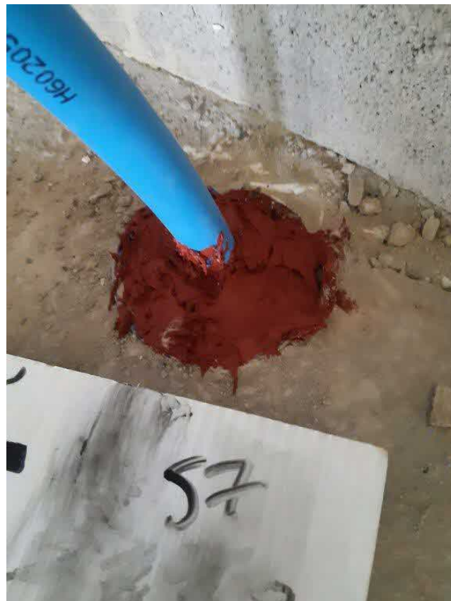
04 C8785E 15.09.23 Plot 57 Service Entry Seal (client photo)
