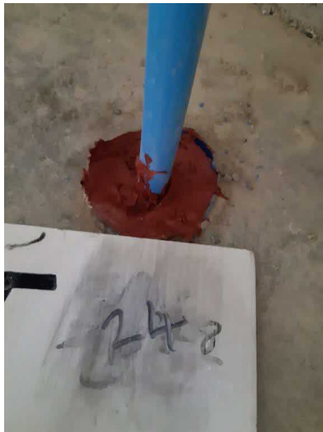
02 C8785E 15.09.23 Plot 24 Service Entry Seal (client photo)
