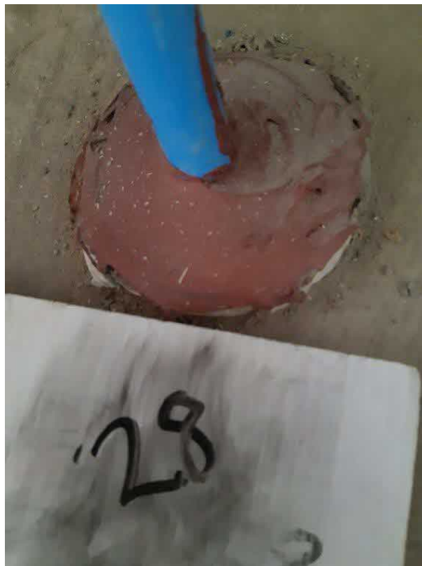
06 C8785E 15.09.23 Plot 28 Service Entry Seal (client photo)
