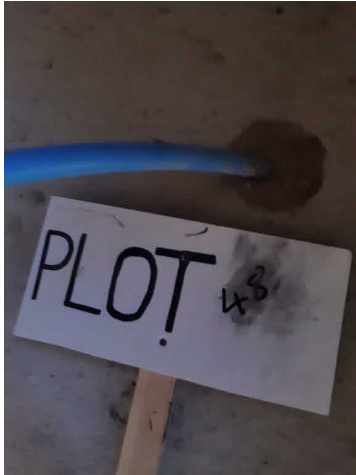
03 C8785E 10.11.23 Plot 48 Service Entry Seal (client photo)
