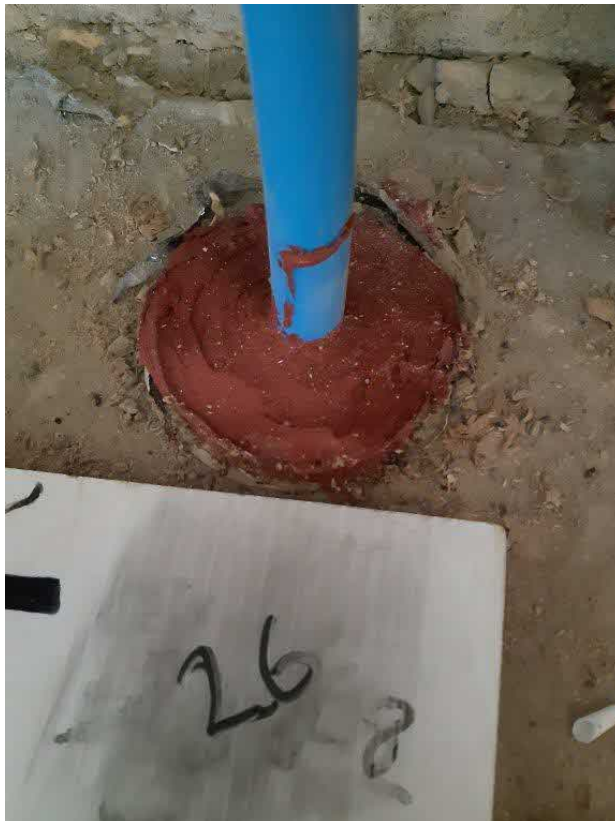
04 C8785E 15.09.23 Plot 26 Service Entry Seal (client photo)
