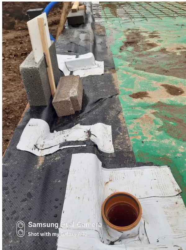
02 C8785E 29.03.23 Plot 55 Corners and Service Entry Duct (client photo)
