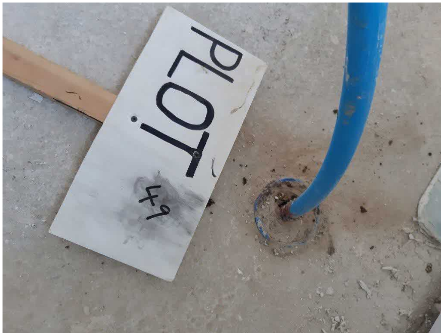
04 C8785E 10.11.23 Plot 49 Service Entry Seal (client photo)
