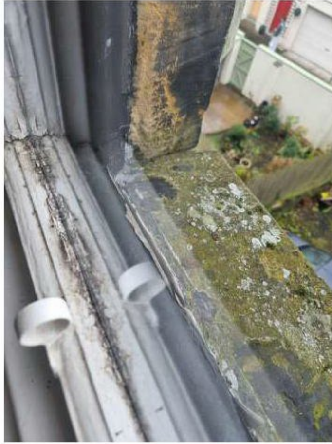
Photo shows deteriorating internal woodwork. The exterior sill is also bare and showing signs of rot. Mastic to the bottom of the casement is no longer present which is allowing water to penetrate the woodwork.
