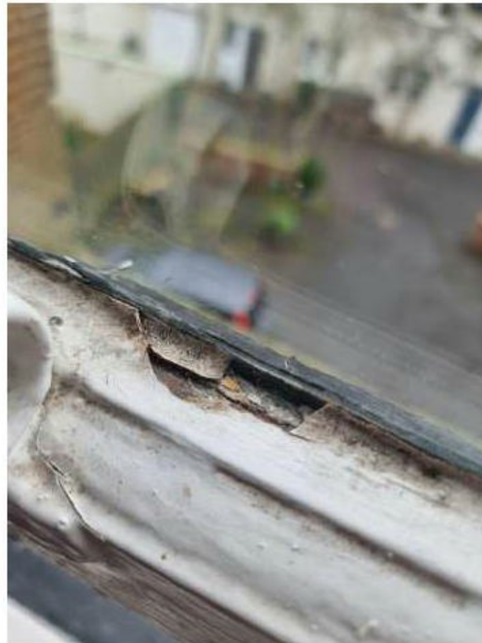
Seals are coming away from the glass.
