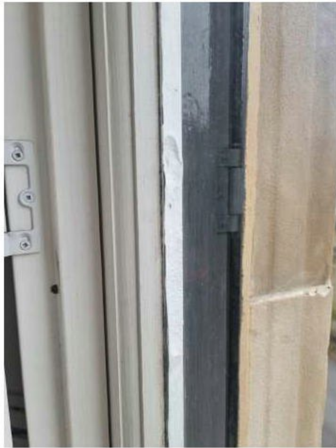
The bottom sashes appear to have already been replaced on two of the windows on the front elevation.
