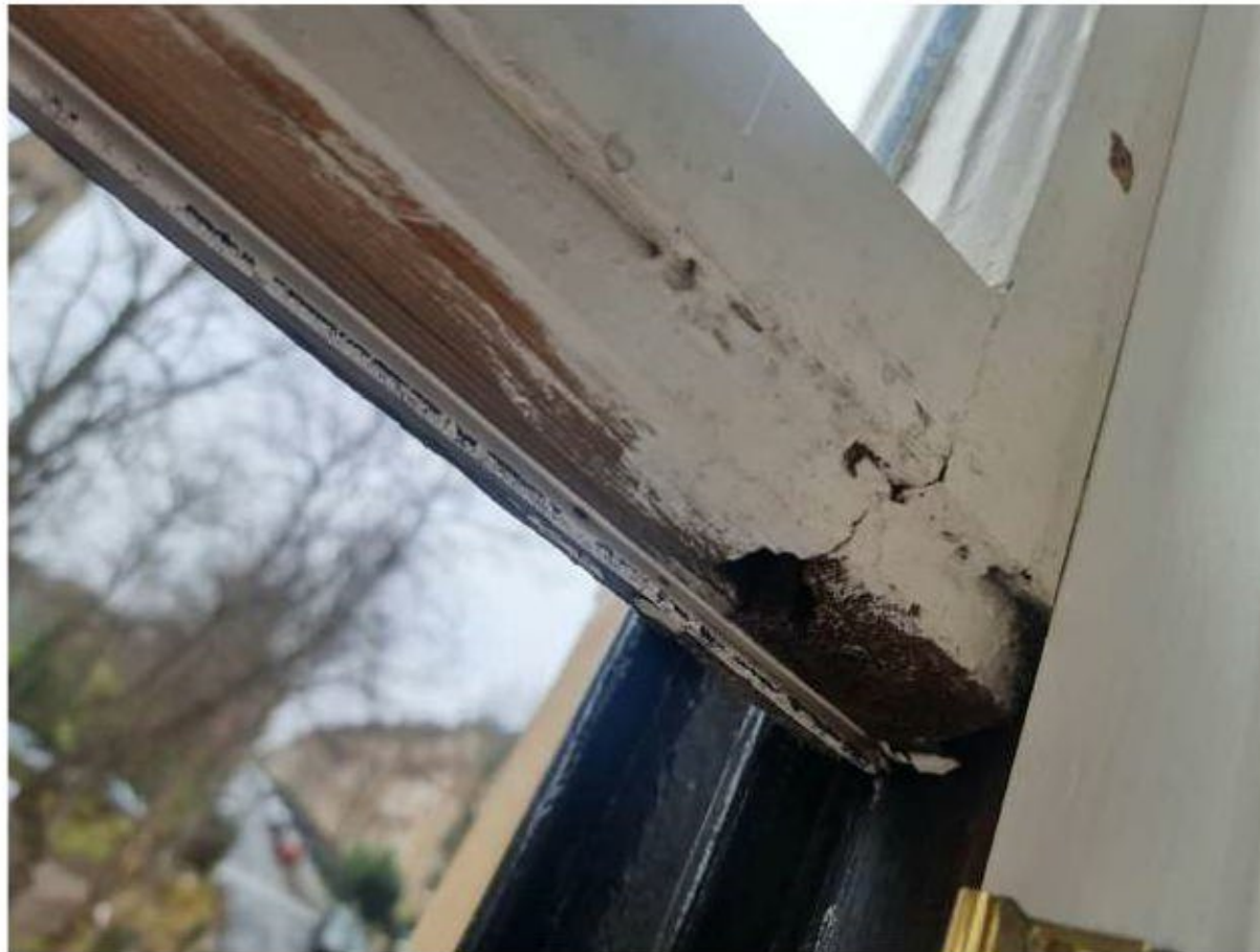
Tenon joint is failing and rotting.
