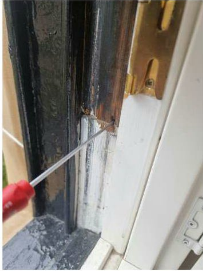
Rotting pulley pocket and casement woodwork.
