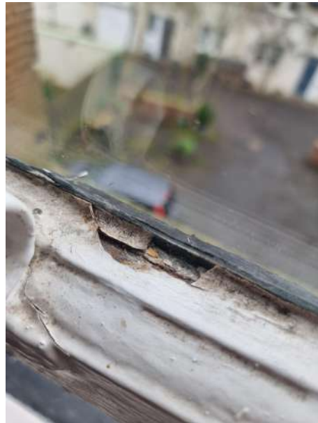
Seals are coming away from the glass.
