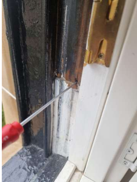
Rotting pulley pocket and casement woodwork.
