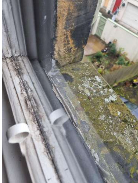
Photo shows deteriorating internal woodwork. The exterior sill is also bare and showing signs of rot. Mastic to the bottom of the casement is no longer present which is allowing water to penetrate the woodwork.
