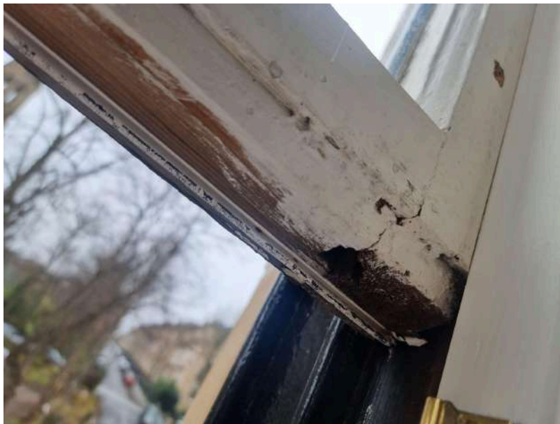
Tenon joint is failing and rotting.
