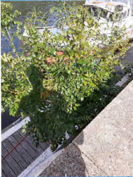
25 – Possible Willow tree growing into quay wall
