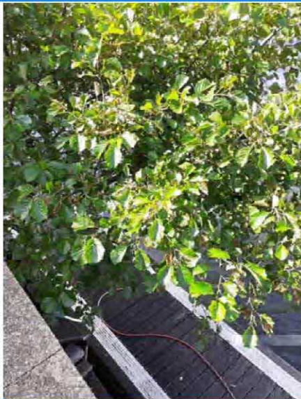
23 – Possible Alder tree growing into quay wall
