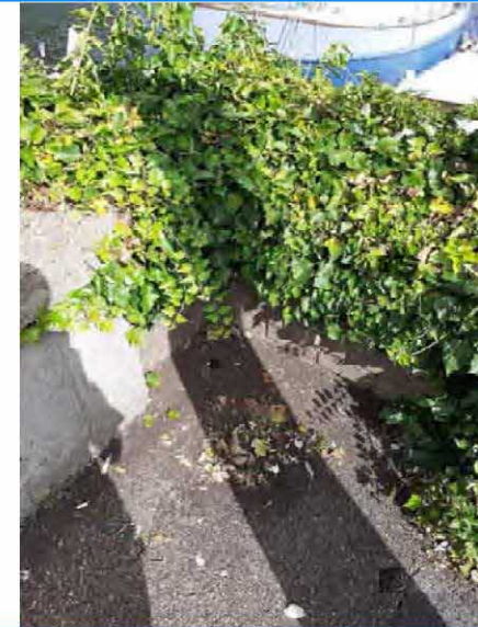
30 – Potentially blocked drain, looking south west
