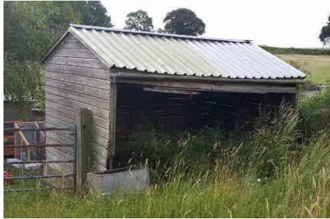
Field shelter at the western end of the row of stables, to remain unaltered and enhanced for use by Swallows.
