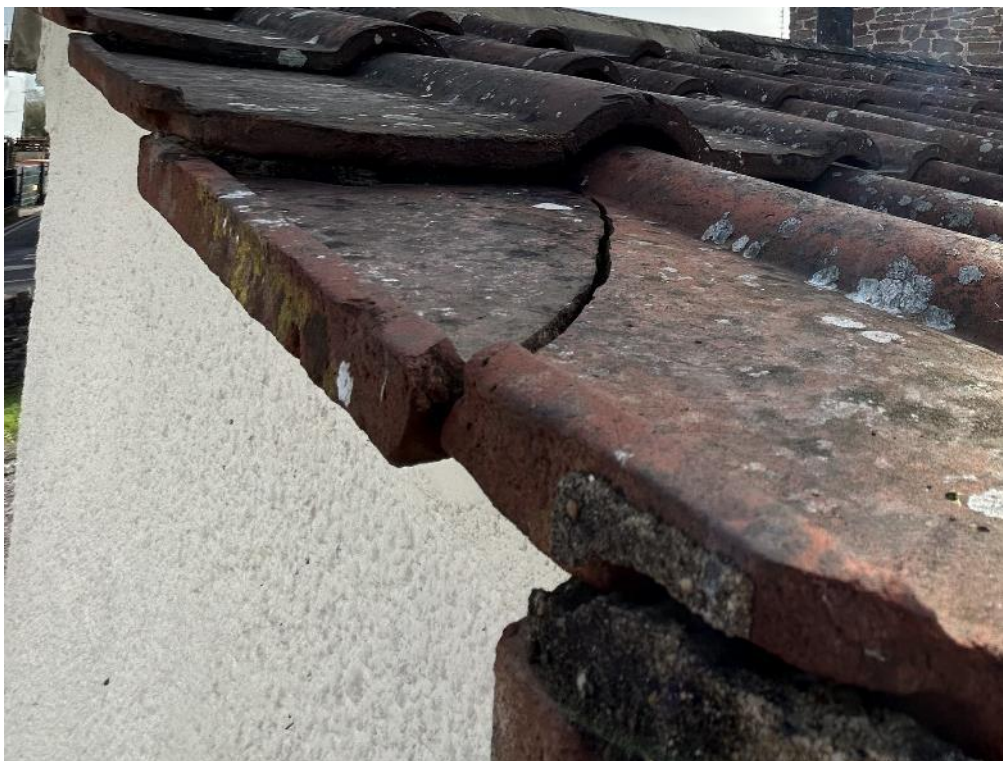
Photograph 22: B1, cracked tile, gently lifted, no evidence of bats
