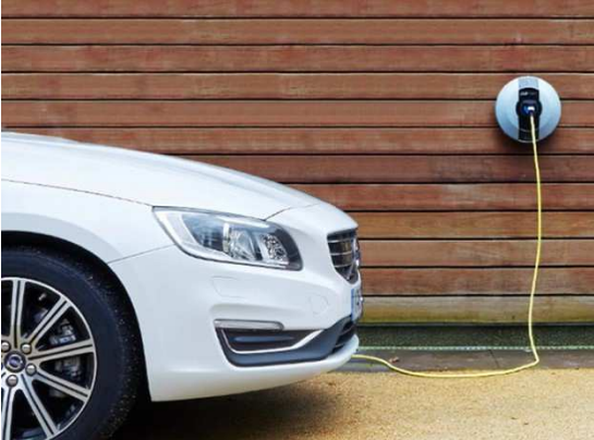
Electric Car Charging Points
