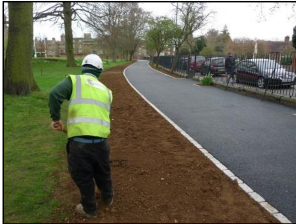
Fig 12 – All 'making good' topsoil will be BS3882 compliant and raked out by hand to no greater depth than 100mm. The garden areas can then be turfed/ mulched/ planted as required.
