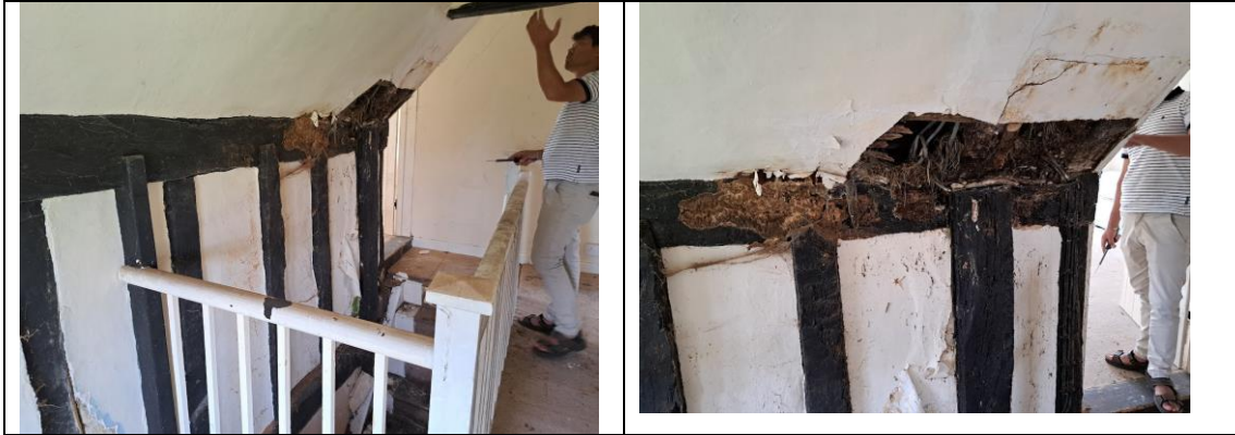
c) Rainwater ingress at base of valley. Wall plate/rafters/post decayed.
