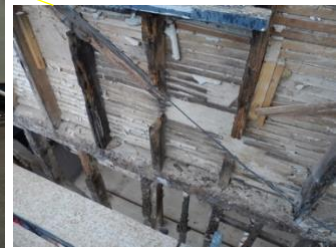
rotting frame under window
