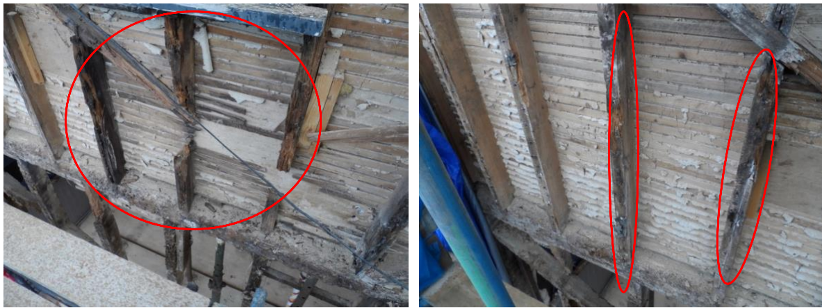
Sections of modern framing below and left of FF window to be replaced using soft wood.
