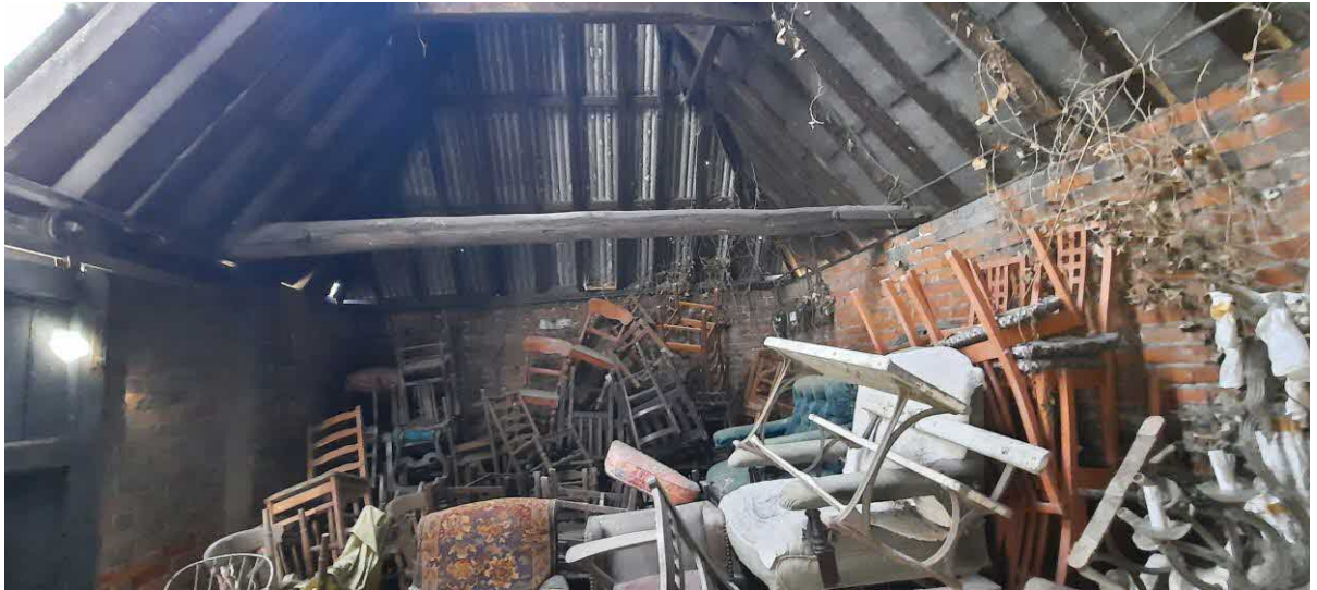
Fig.9 – part of the Forge interior with the front doors evident on the left of the photograph
