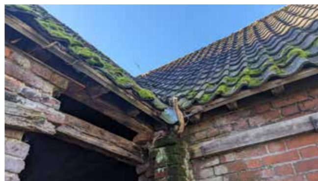
OPENING TO SIDE OF EARLY FORGE, WITH APPARENT TIMBER LINTEL (ROTTEN BEYOND REPAIR)
