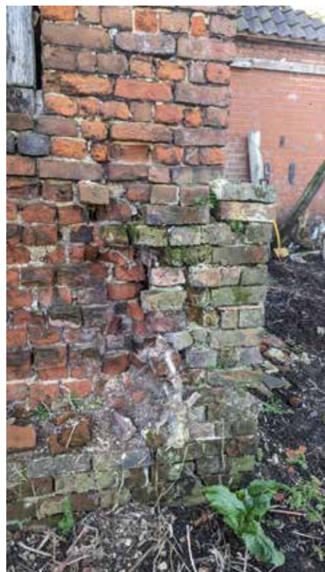
EARLY FORGE DAMAGED AND MISSING BRICKS TO PLINTH.
