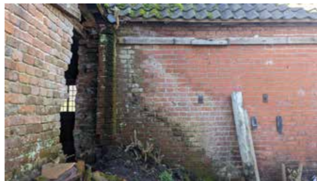
EARLY FORGE SIDE OPENING, WITH DIRT MOUND. TIMBER TO LEAN TO FIXED TO WALL.
