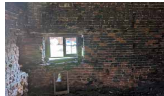
EARLY FORGE CASEMENT WINDOW (DAMAGED)
