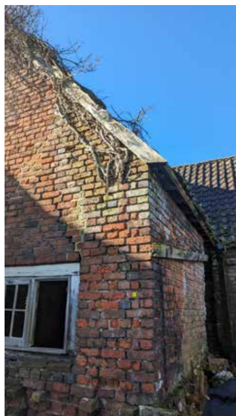
EARLY FORGE'S REAR GABLE, DAMAGED BRICK AND INVASIVE FOLIAGE
