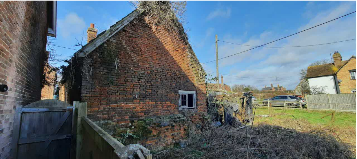
Fig. 5 – the rear (east) elevation of The Forge with collapsed lean-to/outshot
