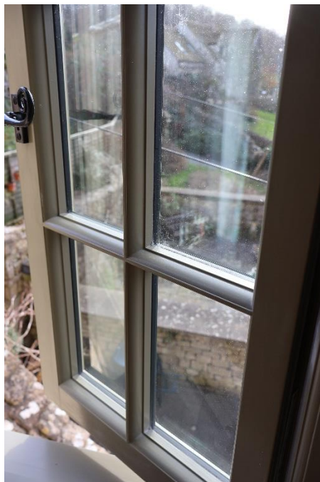
Photograph 6: Detail of internal finish with traditional glazing bar mouldings and the traditional monkey tail fittings
