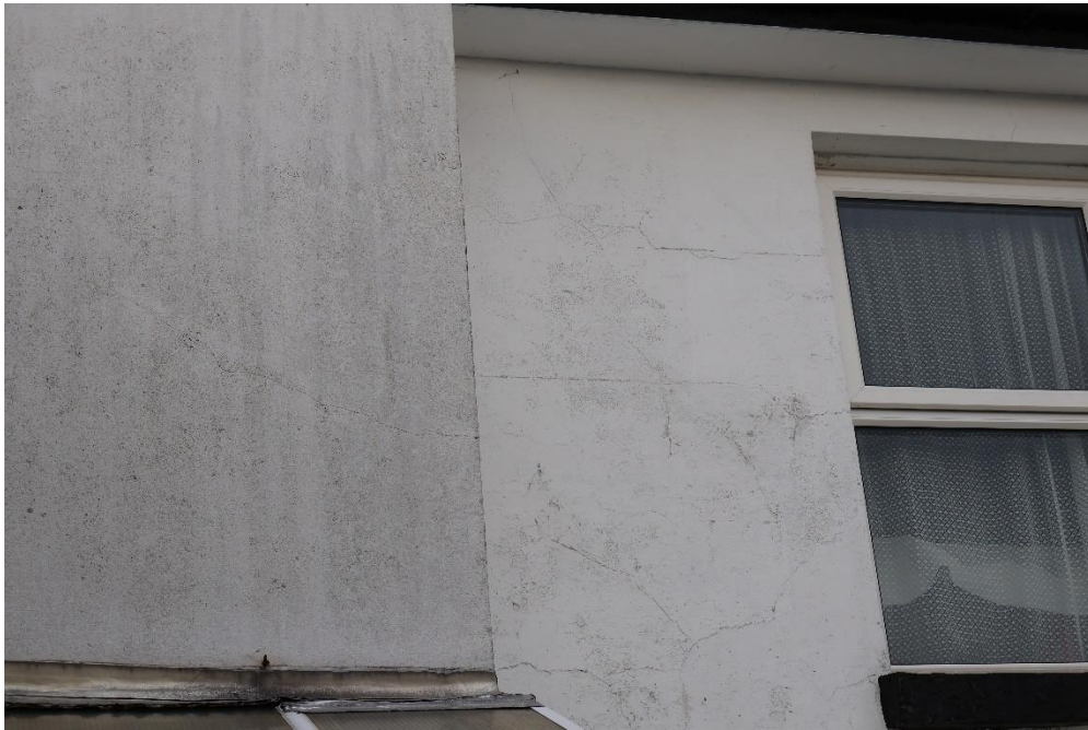
Photograph 2: Rear elevation of 36 and 37 showing the detail of the painted and incised render cladding on the main building contrasting with the later render finish on the rear elevation above the roof of the lean-to of 37 indicating the refurbishment that was undertaken when it was extended. The Upvc window is to be replaced by a timber sash
