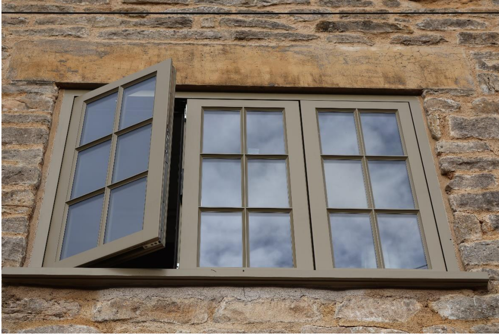
Photograph 5: A three light, timber slim-line, double-glazed casement window with true glazing bars and traditional flush finish recently installed (January 2024) with LBC into a Grade II listed building in Gloucestershire
