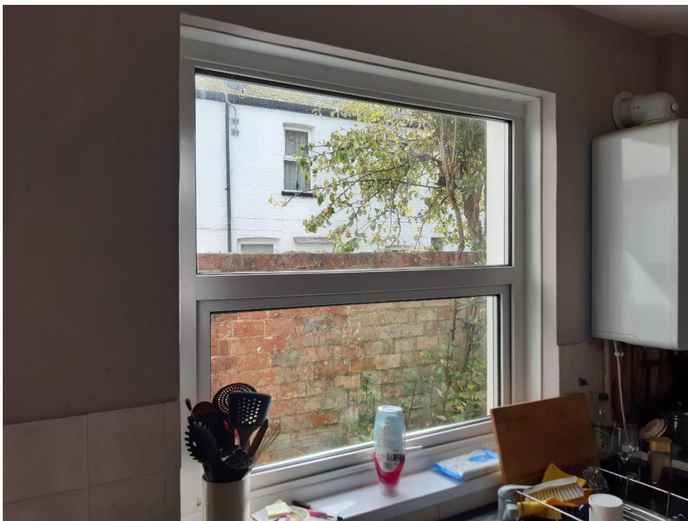
Photograph 3: Rear wing (kitchen) of 37 Upvc window in the east elevation from the inside. It is proposed to replace this window with a two light timber casement.
