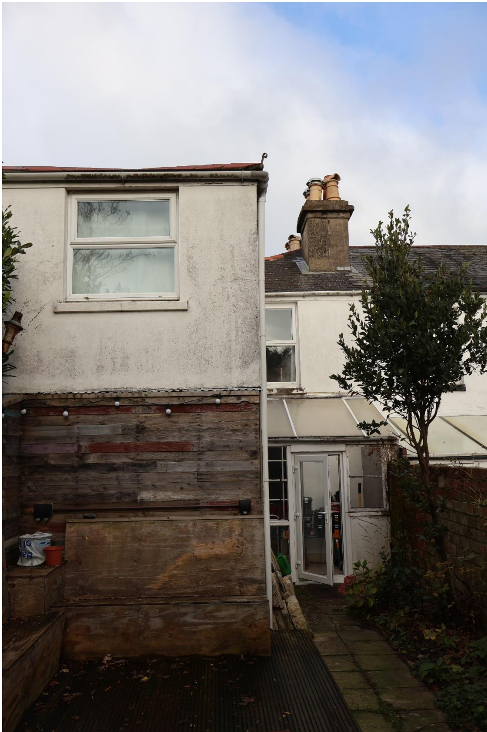
Photograph 1: Rear elevation of main house and later wing from the garden showing the ad-hoc lean to conservatory with a plastic roof and door and the Upvc first floor windows in the south elevation of the main house and the wing .Photograph by the author 2023
