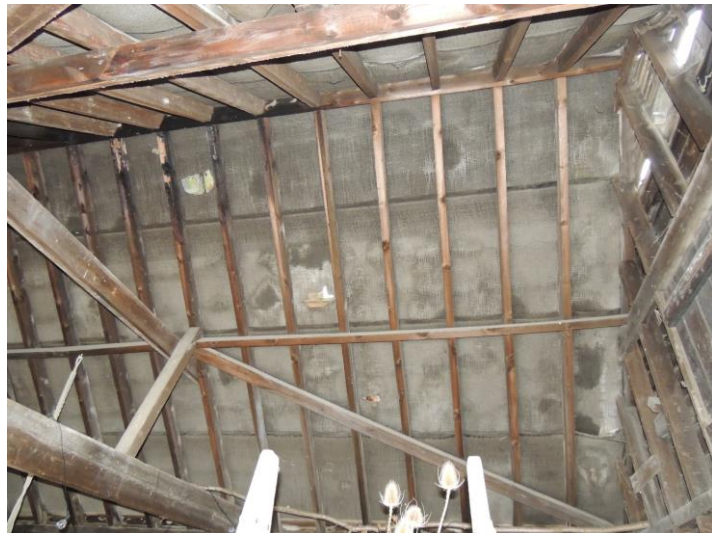
Photo 6: The roof of the cart lodge had no features that might be occupied by bats
