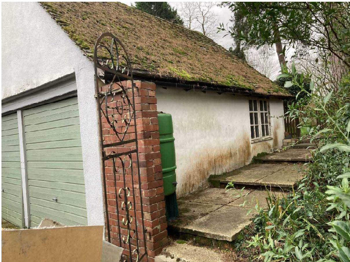
Fig. 3 –View looking south to RHS of existing garage. Note change in ground level.
