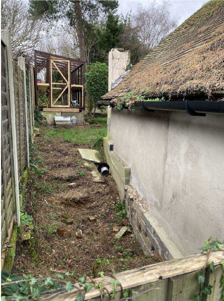
Fig. 6 –View looking south west to LHS of existing garage where new extension is proposed. The changes in height to retaining wall/DPC can be seen on the wall.
