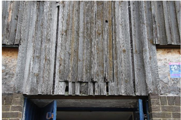
4. Holes in and around southern gable door
