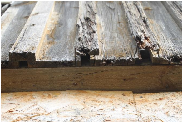
5. Gaps in wooden boarding
