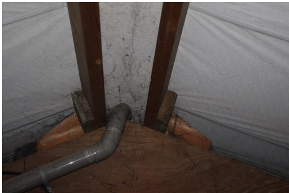
7. Cobwebs in boarded apex
