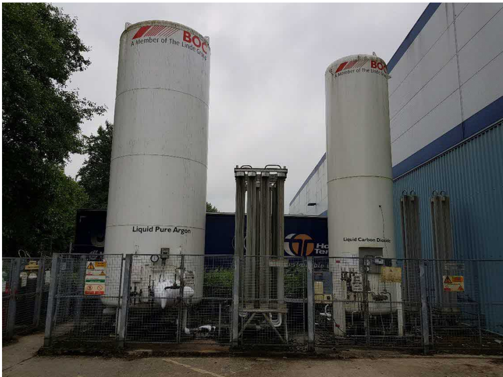
Photo 10: Liquid argon and carbon dioxide tanks, facing SE
