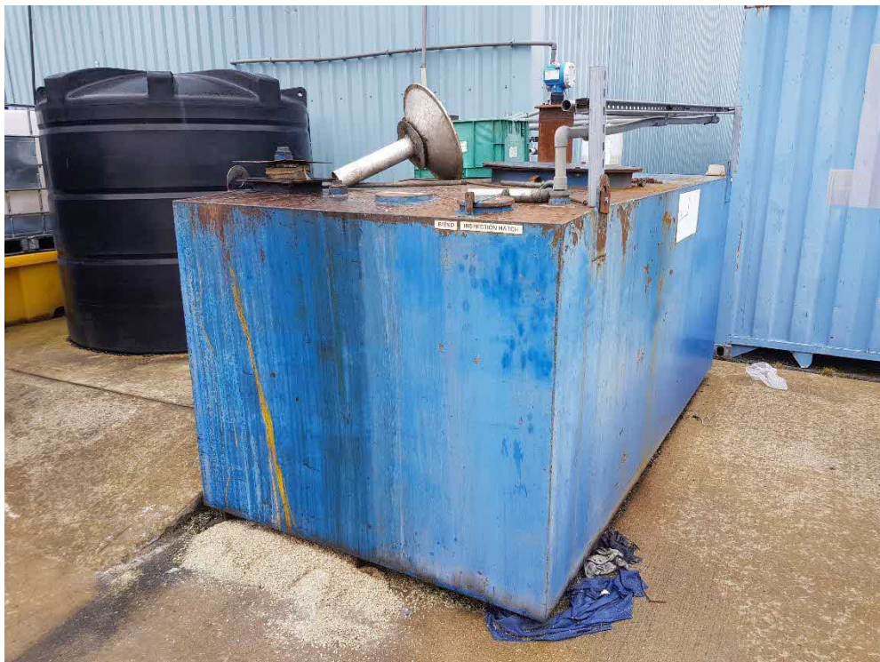
Photo 4: Waste water/oil Above Ground Storage Tank
