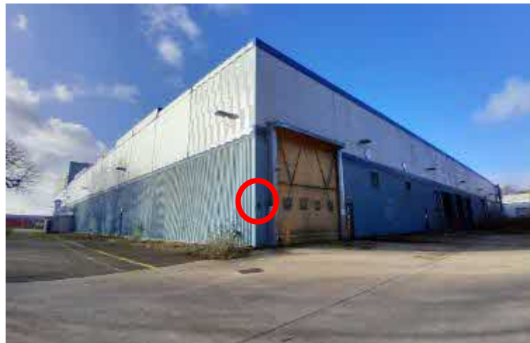
Figure 10 - View of northeast of building 1 with red circle showing location of potential roosting feature.
