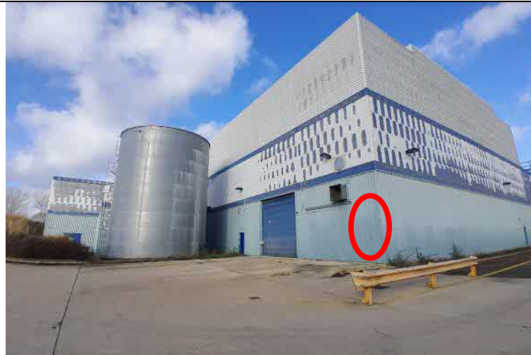
Figure 14 - View of southeastern elevation of building 1 with red circle highlighting location of PRFs.
