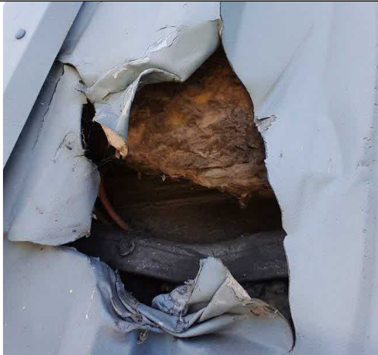
Figure 11 - Close up view of PRF circled in figure 10.
