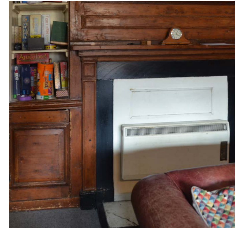
Example of existing direct electric radiator
