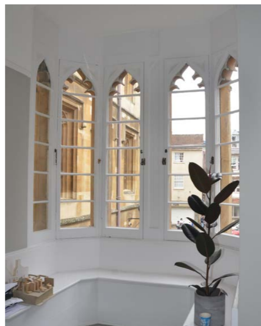
Unsuitable bay window in Bursar's office (T.08)
