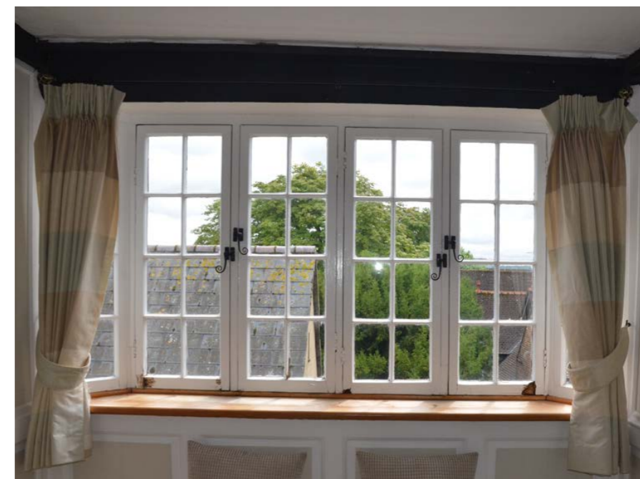
Unsuitable bay window in room 4.6
