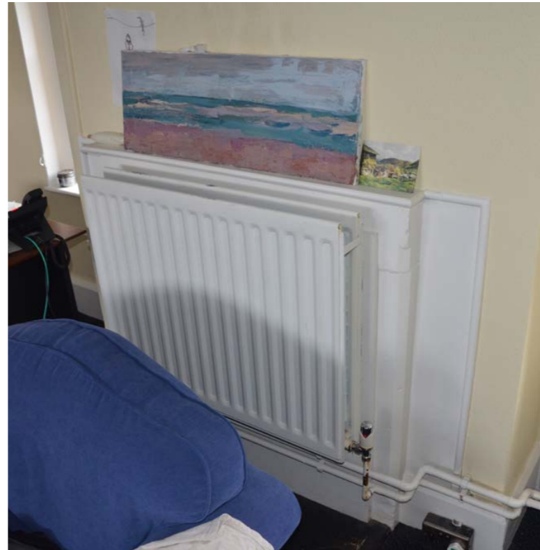
Example of existing water-filled radiator
